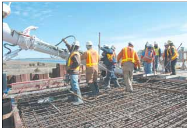
RIGHT: After sliding the new approach span into place, workers pour concrete between the new approach span and the existing roadway.
