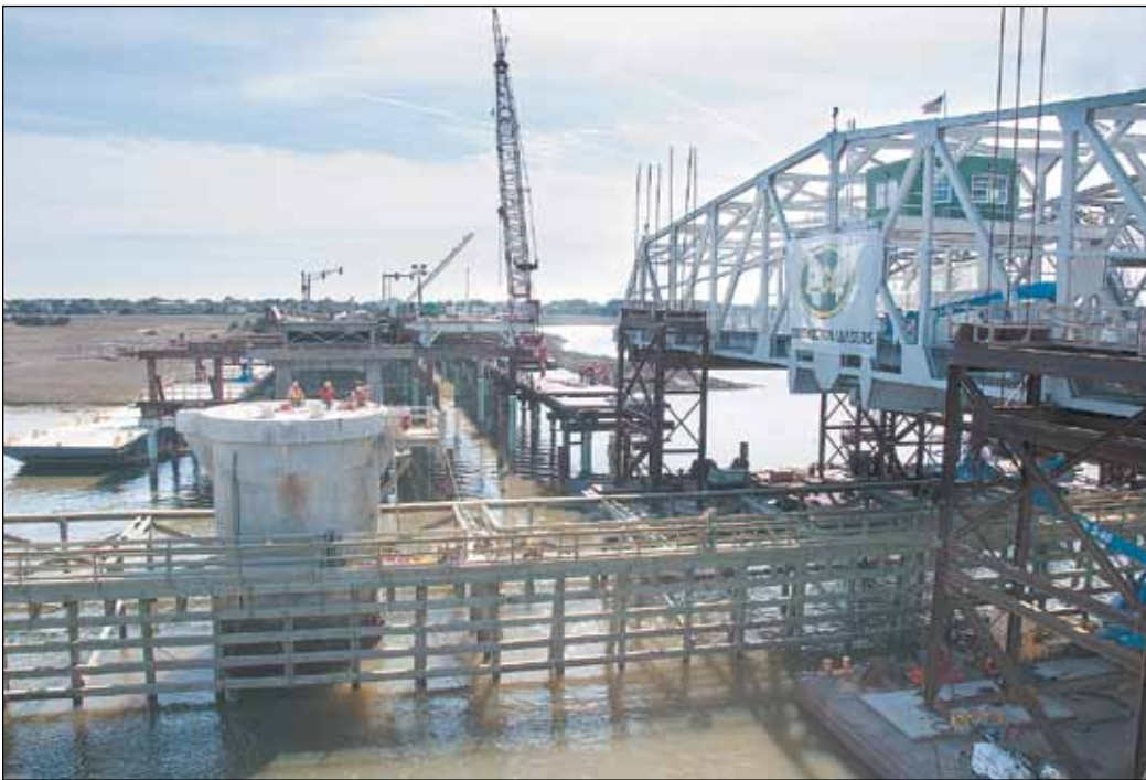
ABOVE: PCL Constructors employees put the finishing touches on the center support where the new swing bridge will rotate to open for boat traffic.
