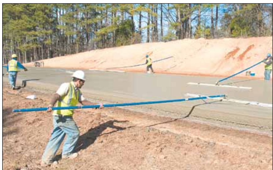
Workers smooth out the 10-inch concrete surface after the GPS paver forms the roadway. After the concrete dries, a pattern is cut into the surface to improve tire grip.
