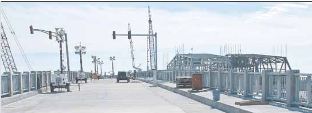
BELOW: The new approach span has new traffic lights, wider travel lanes and a wider pedestrian sidewalk on the harbour side.
