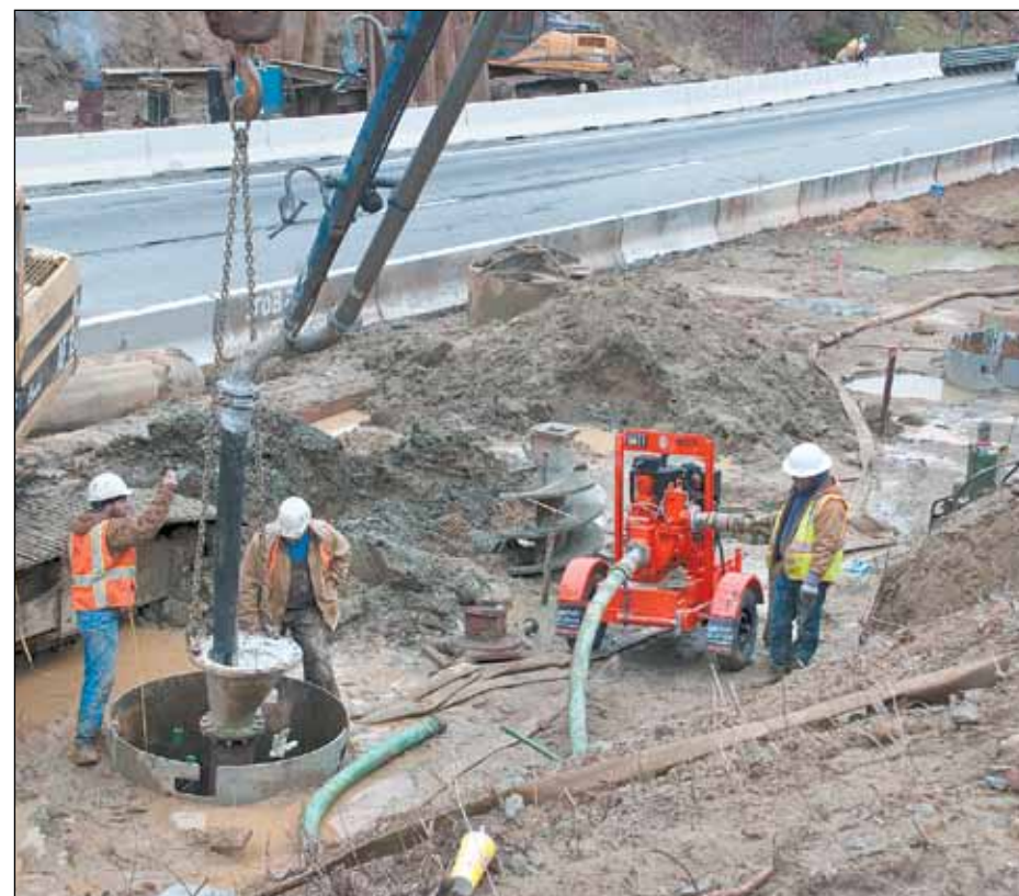
The I-385 flyover bridge over I-26 East has been removed. A pump truck is filling the drill shafts of one of the new bridge's pilings.
