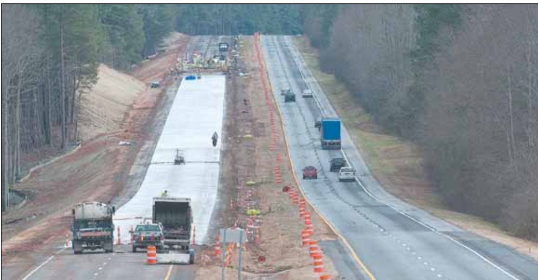
A 15-mile stretch of I-385 North has been closed for a rehabilitation project. The closed portion has been milled and readied for concrete paving. Concrete paving has started on a portion of the closed roadway.
