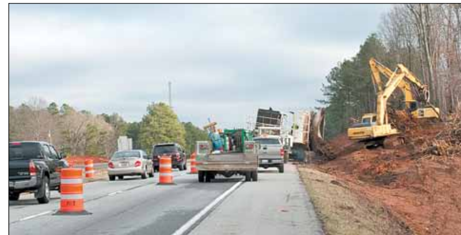
Grubbing and shoulder work is being done on the southbound lanes. Once the northbound work is completed, southbound traffic will be re-routed south down the finished northbound lanes. Rehabilitation work and paving will then be done on the southbound lanes.
