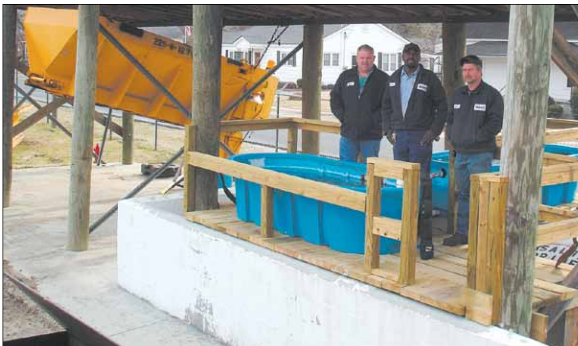
Darlington Maintenance upgraded the platform around their brine tank system recently to make it safer for employees to operate and inspect the process. The mezzanine system is nearly complete, awaiting finishing touches, and it will be ready for the next snow or ice storm. Wayne Locklair, Alphonso Solomon, and Danny Coleman built the brine system in Darlington.
