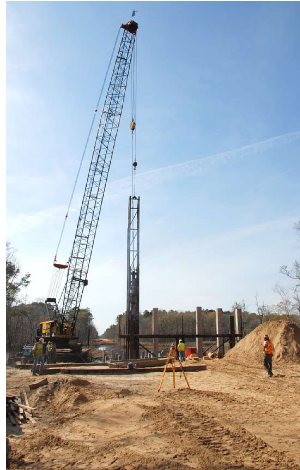
Workers drive pilings for a new bridge that will cross a wetlands area as part of the project.
