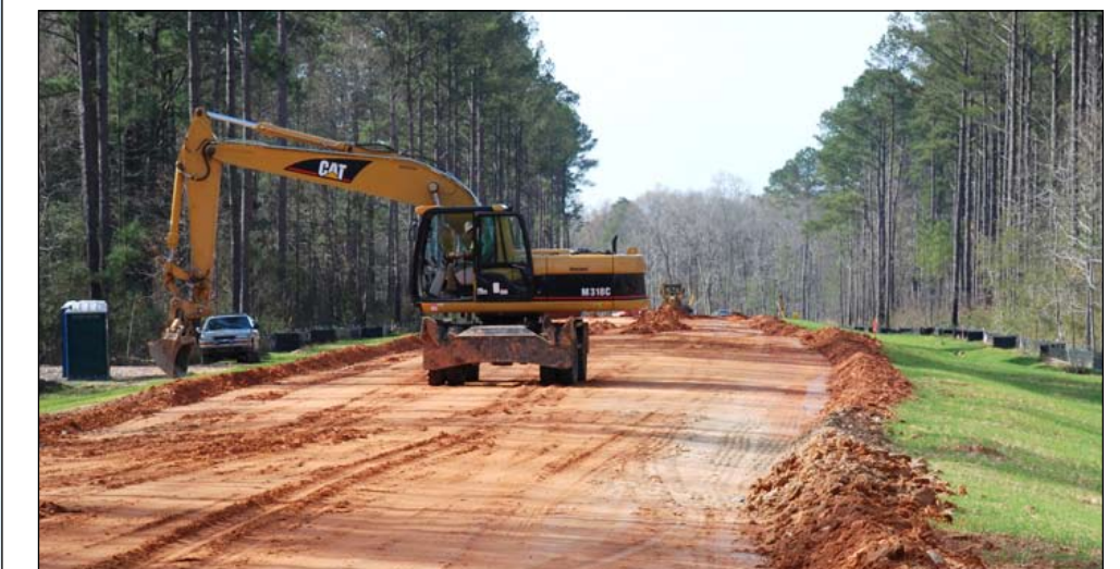
A 70-foot path is being cleared through the area for two 12-foot lanes and 10-foot shoulders.
