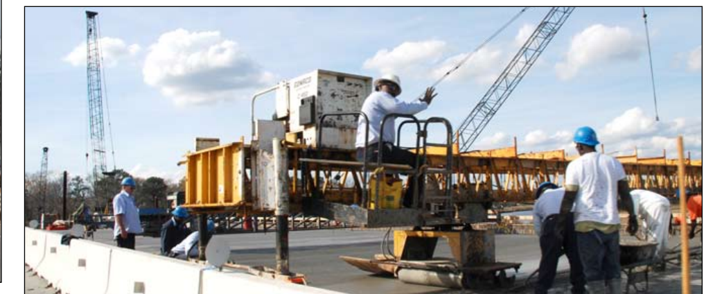
Workers pave the bridge deck of the new bridge being built on US 17 over the Combahee River.
