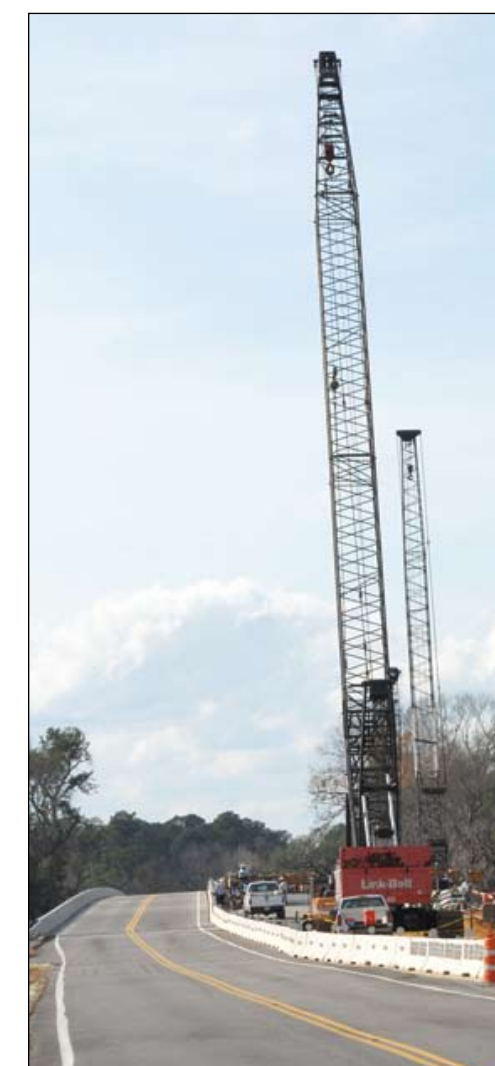
The widening of US 17 included the construction of a new bridge over the Combahee River.
