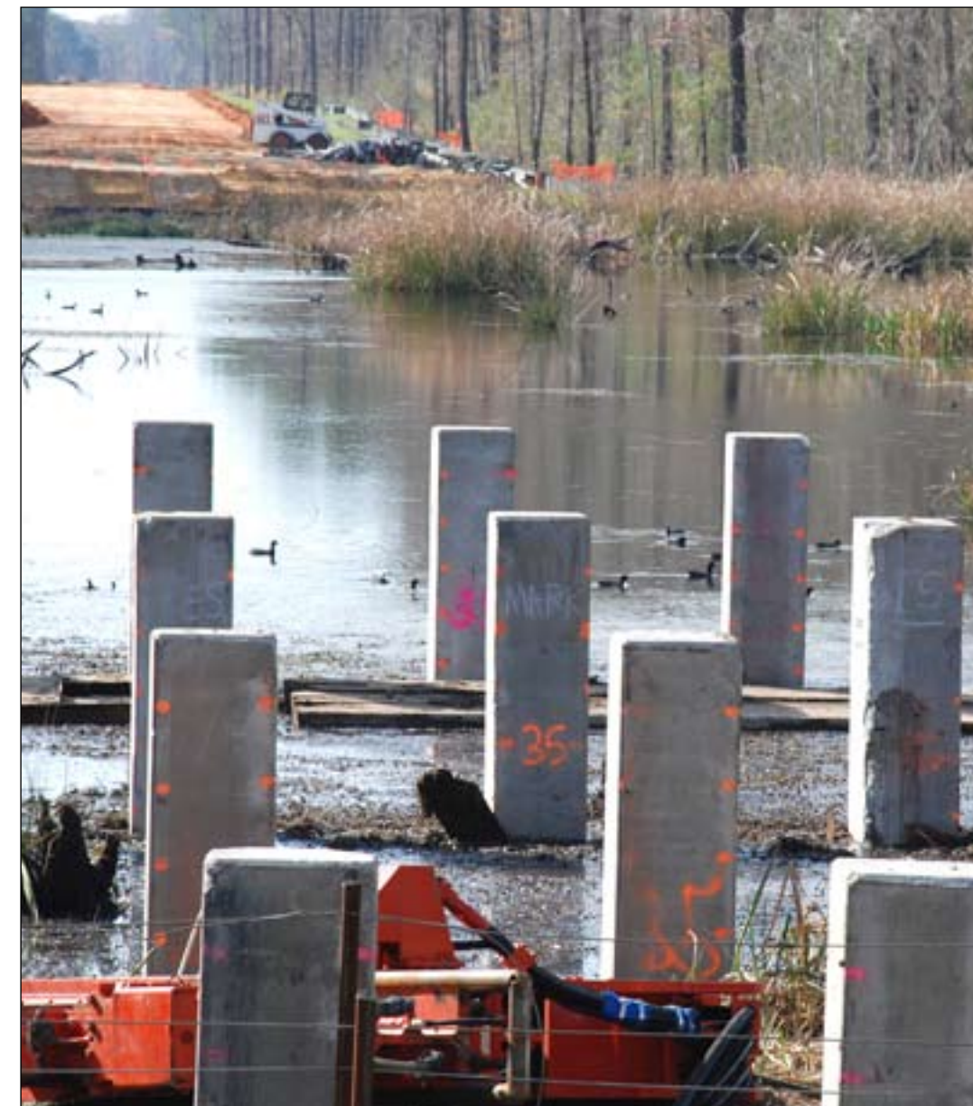
Even as pilings are driven into the river bed, ducks swim past the project.
