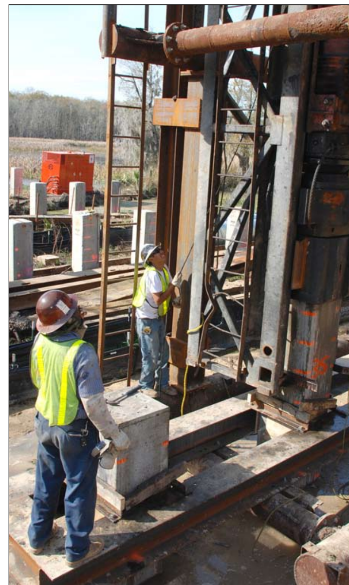
Workers make adjustments to the pile driver as it drives a piling 40 feet into the ground.
