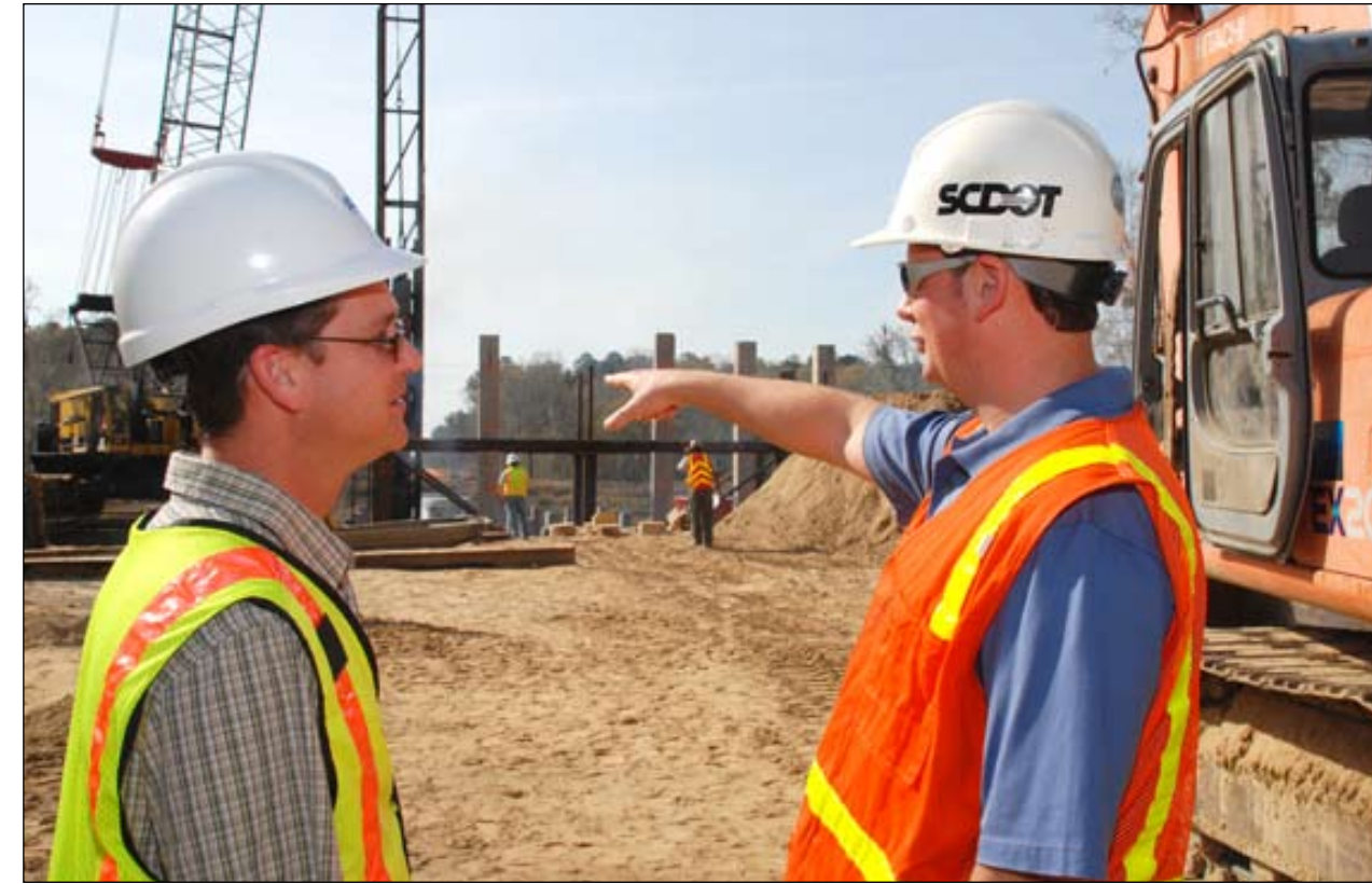
SCDOT Project Manager Chris Hernandez and HDR Project Manager Dennis Meder inspect the pile driving on the project.
