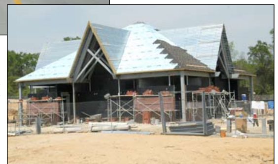
RIGHT: New rest areas are under construction on I-20 in Kershaw County. The new facilities will replace buildings built in 1983. The new facilities are scheduled to open later this year.
