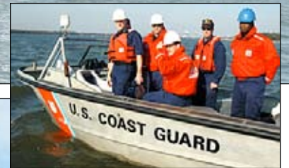
ABOVE: Members of the U.S. Coast Guard watch as the last remaining section of the Grace Bridge over the Cooper River is hauled away on a 350-foot barge March 1. The section was lowered on to the barge by four 900-ton hydraulic strand jacks before being taken to the old naval base where the steel is being recycled.
