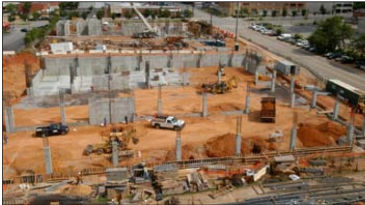
PHOTOGRAPHS BY ROB THOMPSON/THE CONNECTOR Dust particles from construction and demolition work done near SCDOT headquarters can affect air quality in the building. Here, a new hotel is being built in the old SCDOT parking lot north of headquarters.
