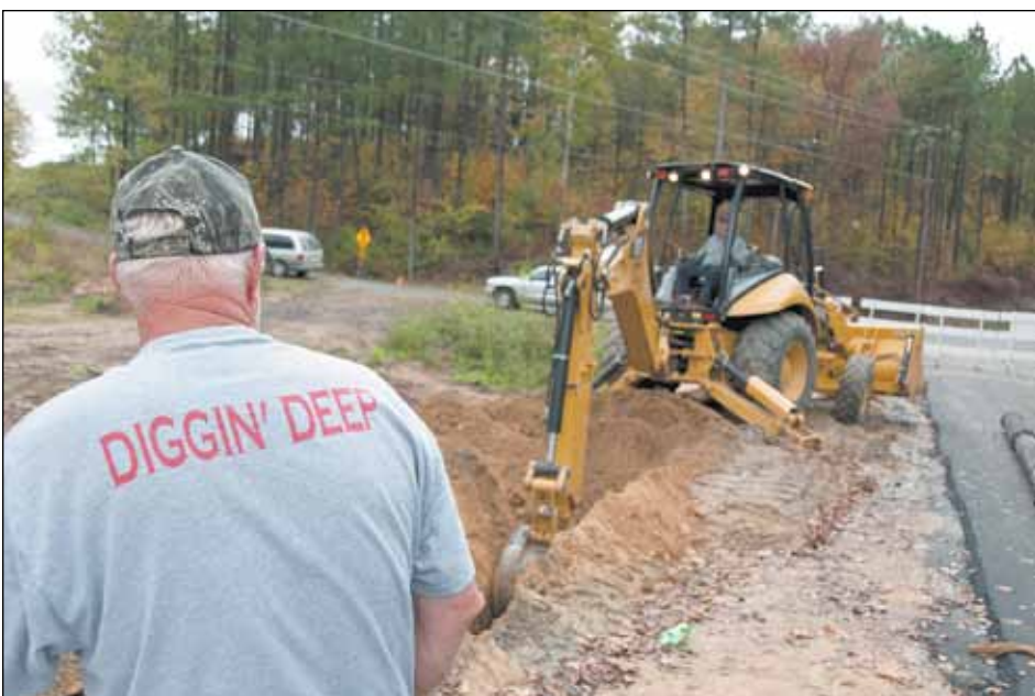
Robert Miller, left, watches as Billy Good digs a trench for a water line along the new bridge. The men work for Good Construction of Great Falls.
