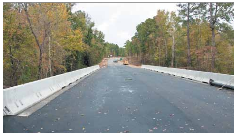
The new Rochelle Creek bridge on River Road is 40 feet longer than the original bridge.
