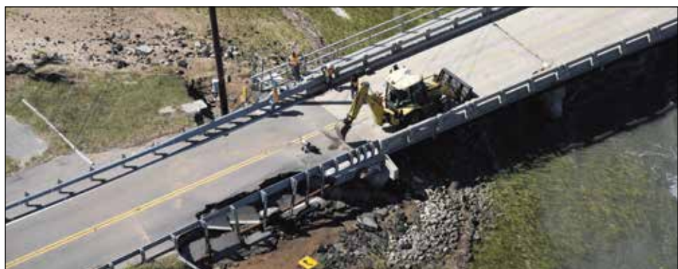
SCDOT crews make repairs to a washout on the Harbor Island Bridge on Oct. 9, 2016.
