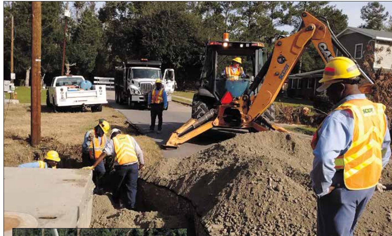
The District 5 Bridge Crew works to repair a washout in Williamsburg County.
