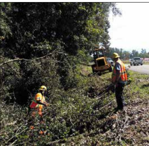
Downed tree removal in Bamberg
