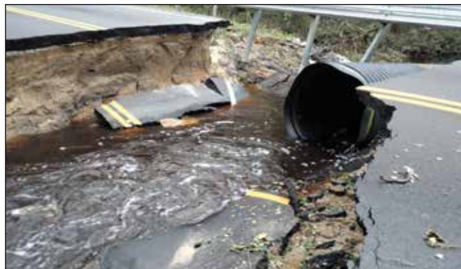
Hurricane Matthew flooding caused a washout on Old Black Oak Road.
