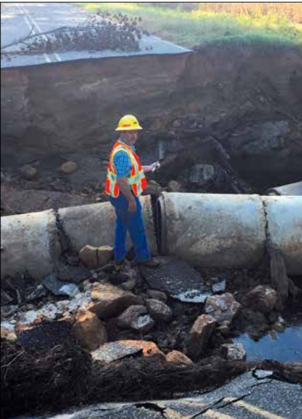
Dillon Maintenance employee Neil Carmichael inspects a washout in Dillon County.
