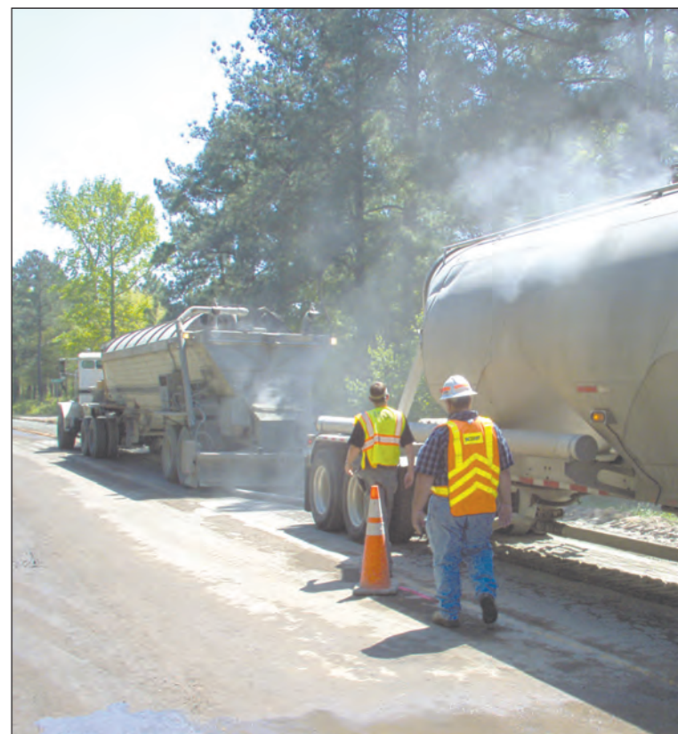
Assistant Resident Construction Engineer Harry Langford checks the reloading of the cement spreader on the reclamation project.
