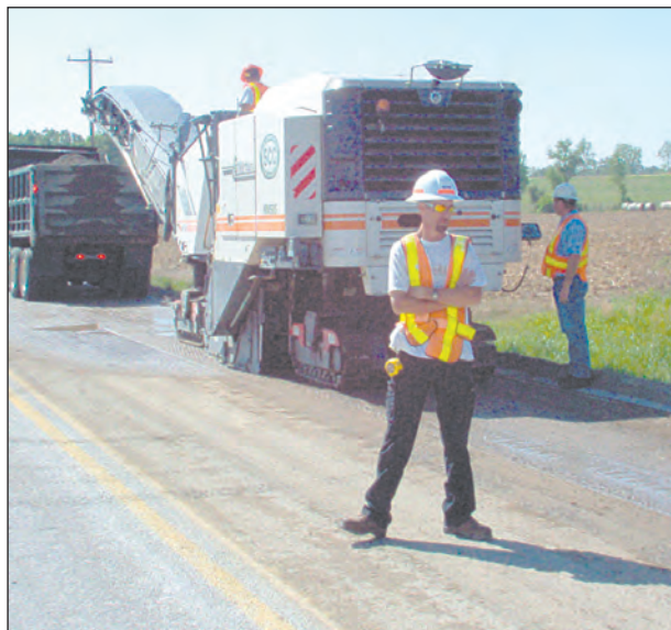
Allen Oxendine monitors the surface planing prior to placing intermediate asphalt on the roadway.
