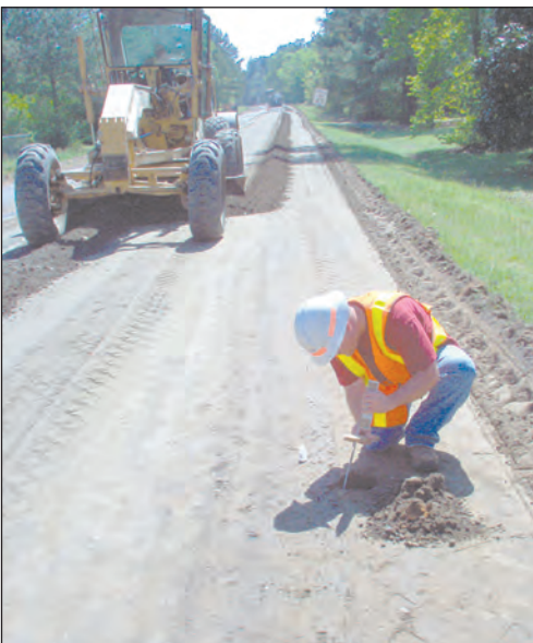
Inspector Jeffrey Taylor does a depth check on the reclaimed base material.
