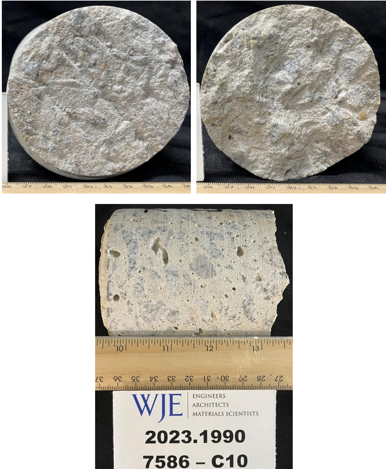
Figure 6. 7586-C10. As-received, with the top surface in the top left image, bottom surface in the top right, and a longitudinal view of the core with the top surface to the left in the bottom image. Note the severely eroded top surface.
