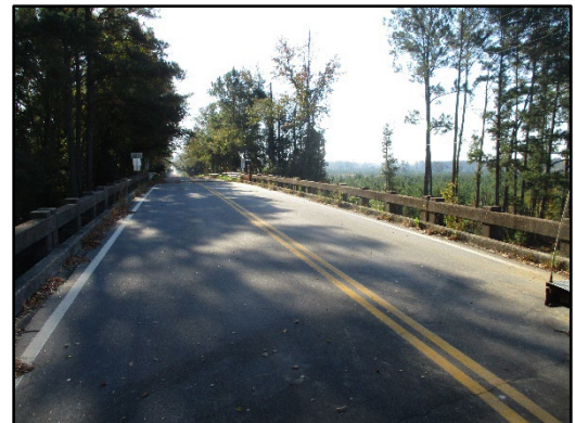
Photo 1: US 21 (Frampton Rd.) RBO CSX Railroad in Hampton and Beaufort Counties, South Carolina.
