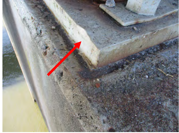
Photo 2. LBP on Bearing Plates Associated with Bridge #3.
