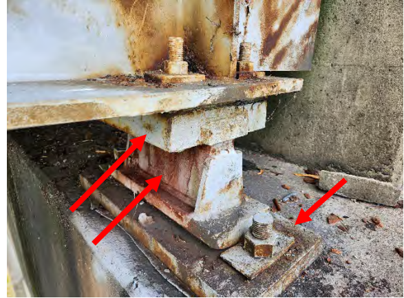
Photo 2. LBP on Rocker Bearing Top Plates, Rocker Bearing and Bearing Plates Associated with Bridge #2.
