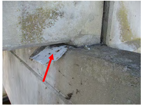
Photo 4. ACM Bond Break Bearing Pad Associated with Bent #28 of I-95 SBL Bridge #3.
