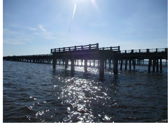
Photo 2. Bridge Remnant on West Side of US 301/15 Trail Bridge over Lake Marion.
