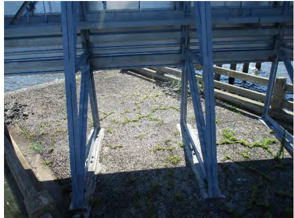
Photo 4. Galvanized Metal Sign Attached to Top of Deck on Bridge Remnant.
