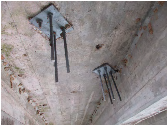
Photo 5. Galvanized Metal Sign Anchor Plates on Underside of Bridge Remnant.
