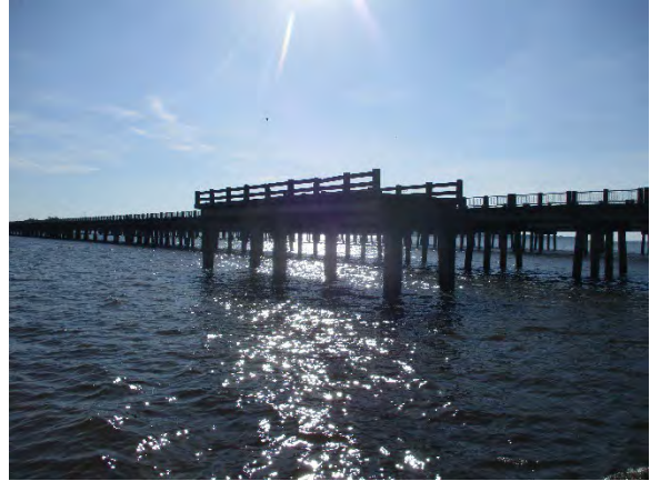
Photo 2. Bridge Remnant on West Side of US 301/15 Trail Bridge over Lake Marion.
