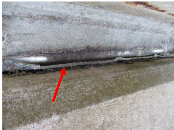
Photo 4. ACM Bond Break Bearing Pad Associated with Bent #28 of I-95 NBL Bridge #2.
