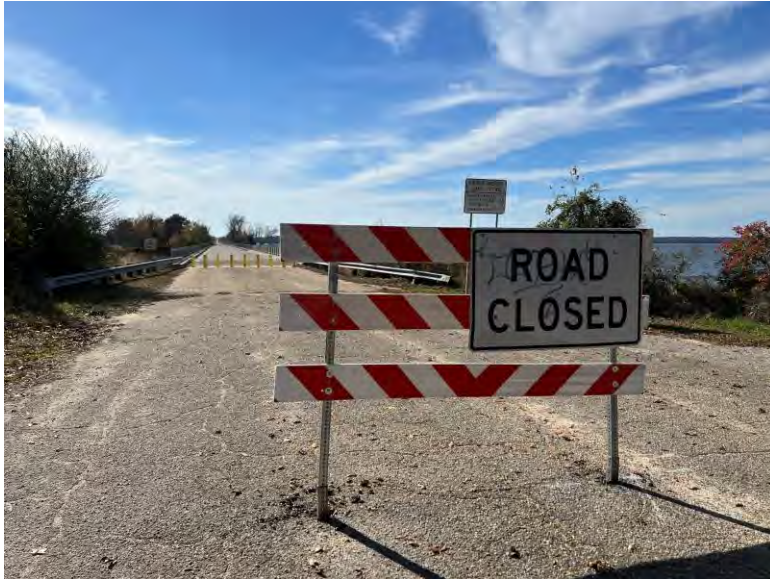
View of the Francis Marion Bridge (formerly US Hwy 301) over Lake Marion from the Summerton side (Clarendon County) within the Project Area.
