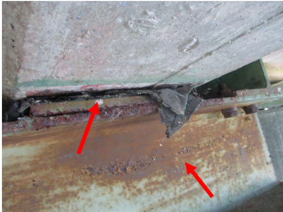
Photo 3. LBP on Gray Repair I Beam and Top Bearing Plate.
