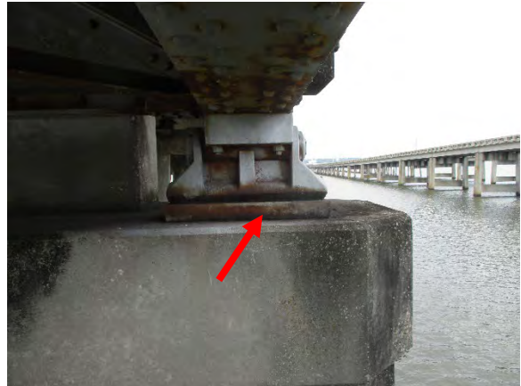
Photo 4. LBP on Gray Bearing Plate under Rocker Bearing on South End of Bridge #6.
