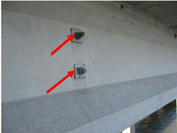
Photo 3. LBP on Tie-Rod Washers Located along each Side of Bridge #3.
