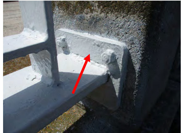
Photo 4. LBP on Gray Metal Handrail Plates along each Side of Bridge #5.
