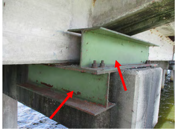
Photo 2. LBP on Green Repair I-Beams Associated with Bridge #6.
