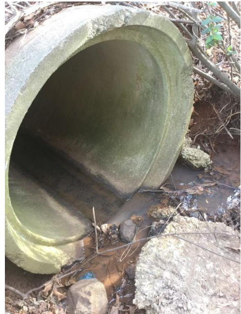
Invert in of Ex. 42" RCP
