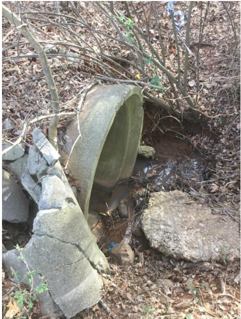
Invert in of Ex. 42" RCP
