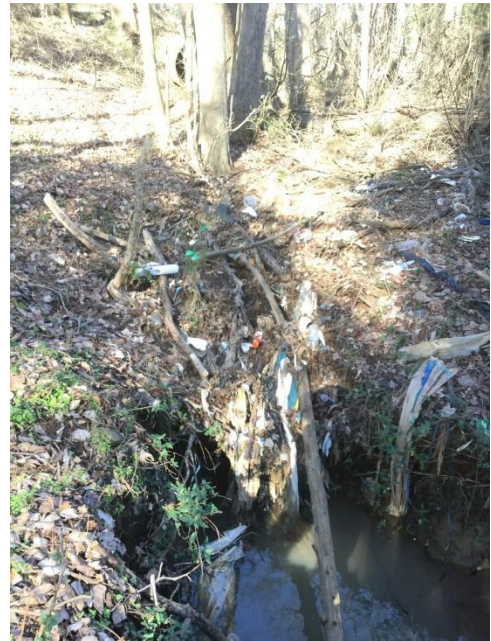
Headcut approx. 50' downstream of Ex 42" RCP looking upstream towards outfall
