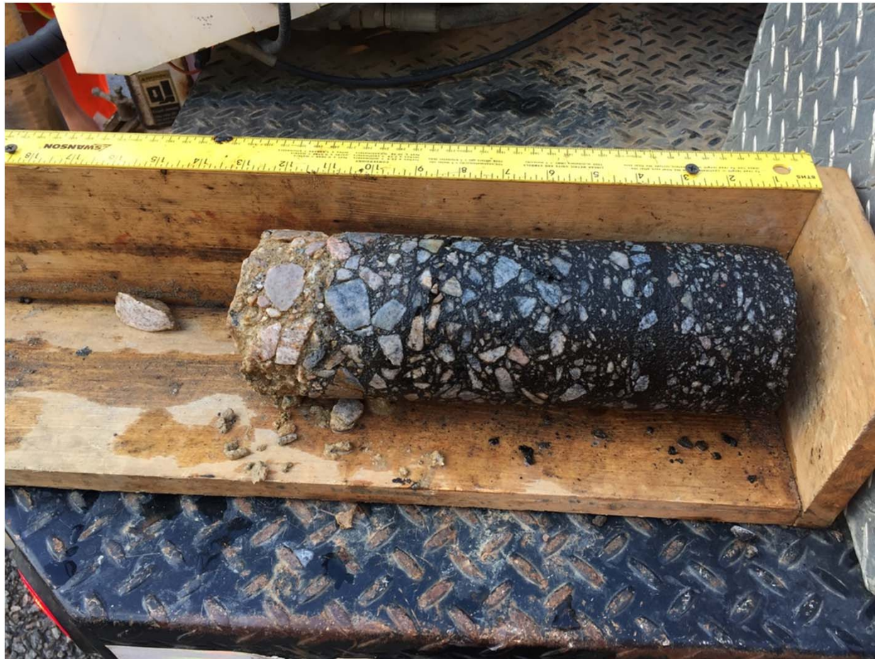
I-26 MM 90.0 eastbound outside lane (a)
