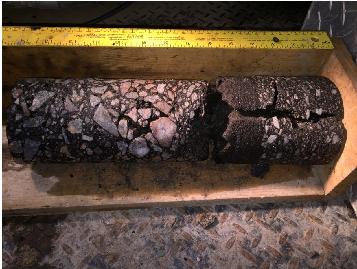
I-26 MM 92.0 eastbound inside lane
