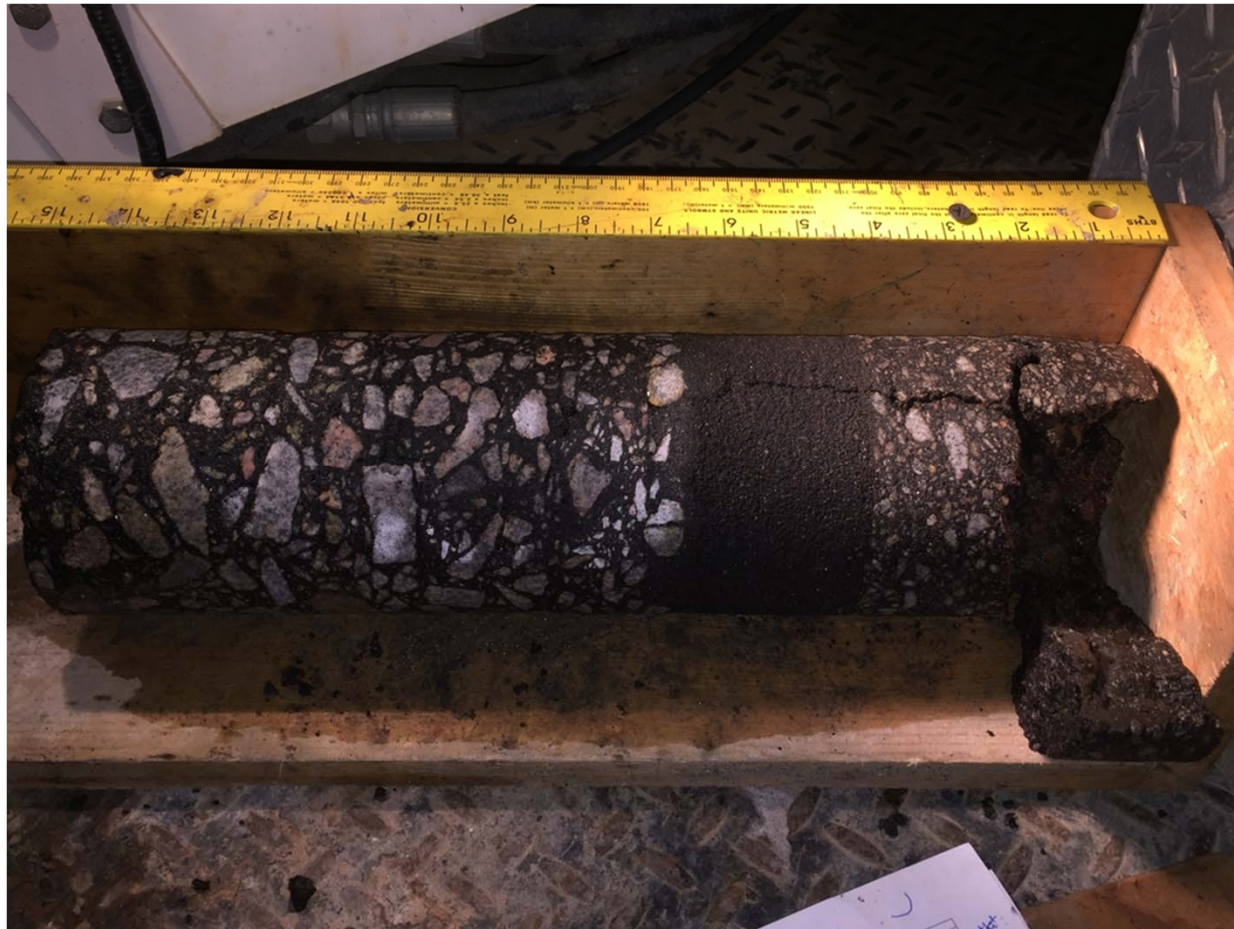
I-26 MM 93.0 eastbound inside lane
