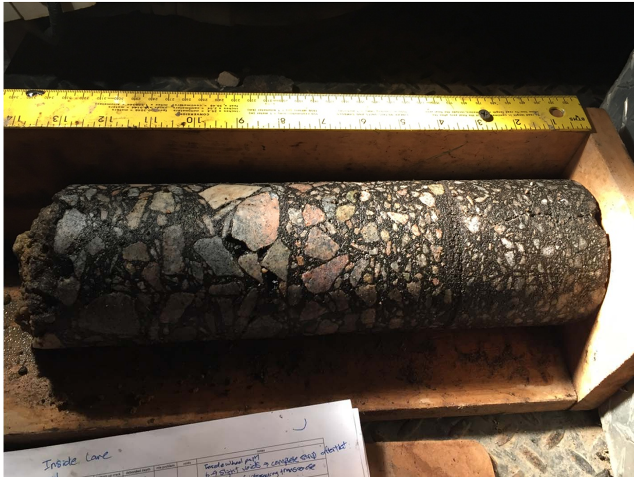
I-26 MM 96.0 eastbound inside lane
