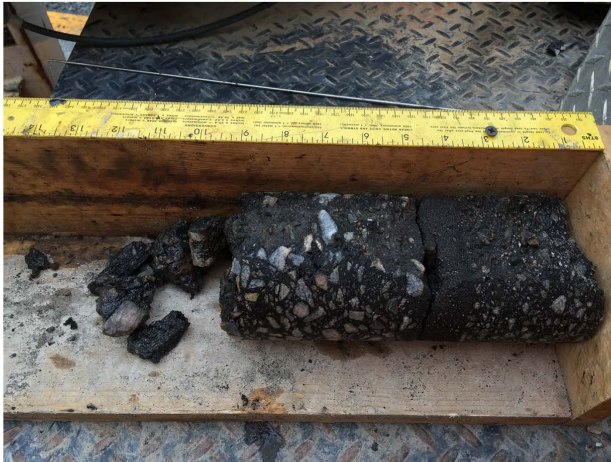
I-26 MM 85.0 eastbound inside lane
