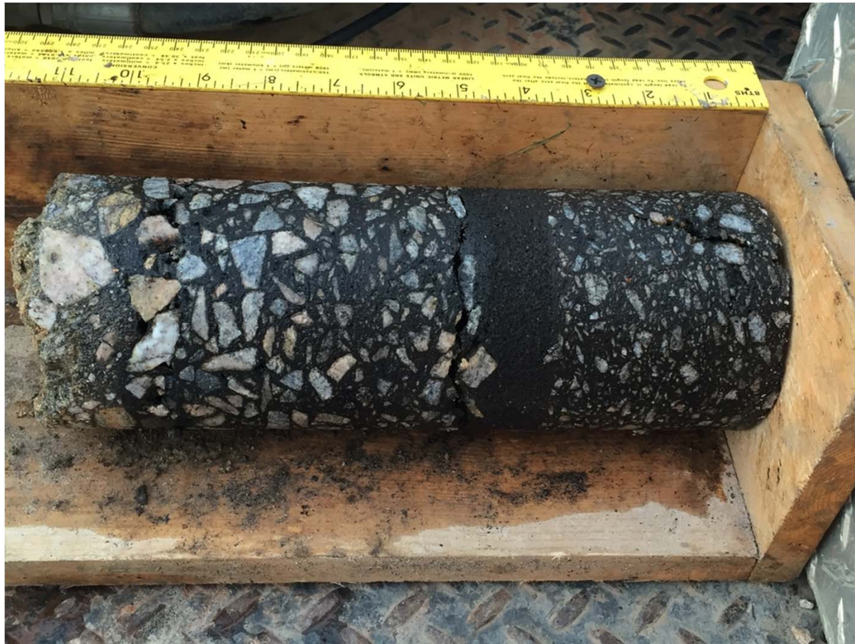
I-26 MM 90.0 eastbound inside lane
