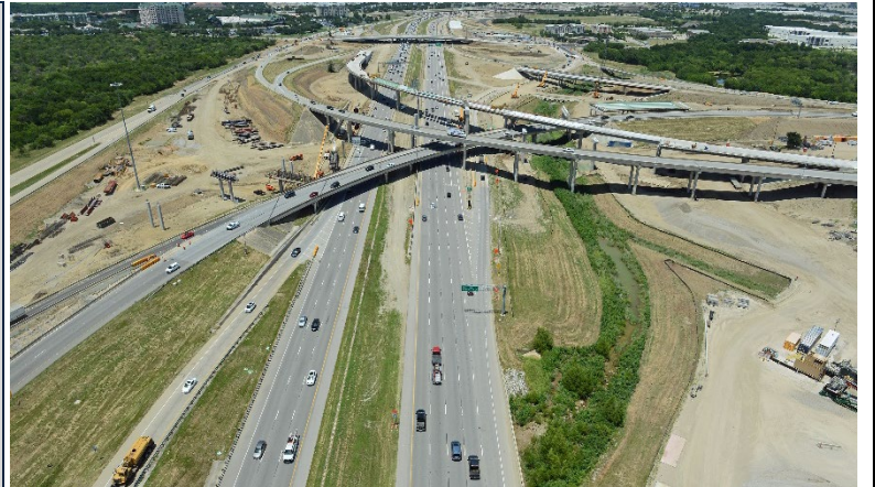
The project required five overpasses and 37 bridges that included two interchanges, five overpasses, and 2,000 girders
