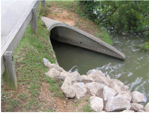
Use Pipe Flared End Section when specified in the plans or special provisions.
