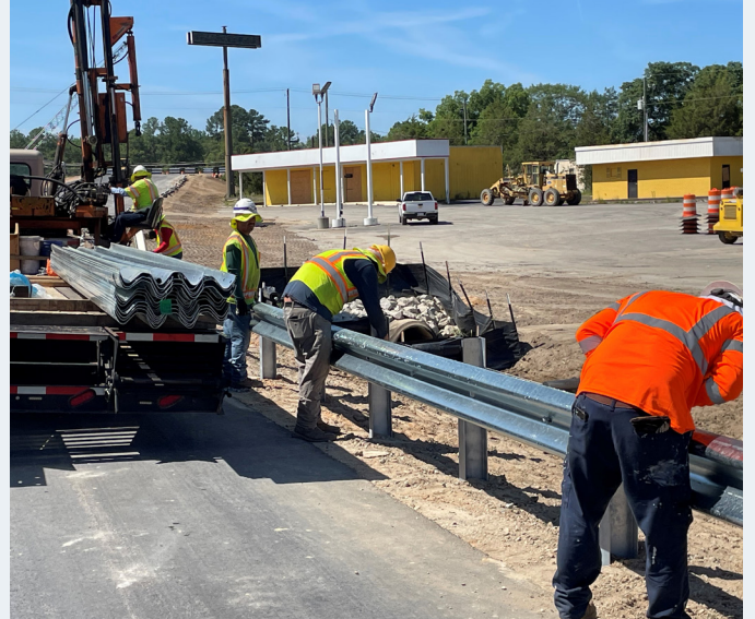
Crew from Reynolds Fence and Guardrail install new guardrail at I-26 approaching the St. Matthews exit, 119.
