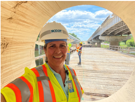
Mary Wyeth and Leila Kelly on-site at I-20 Bridge Replacements over Wateree River (Kershaw County).
