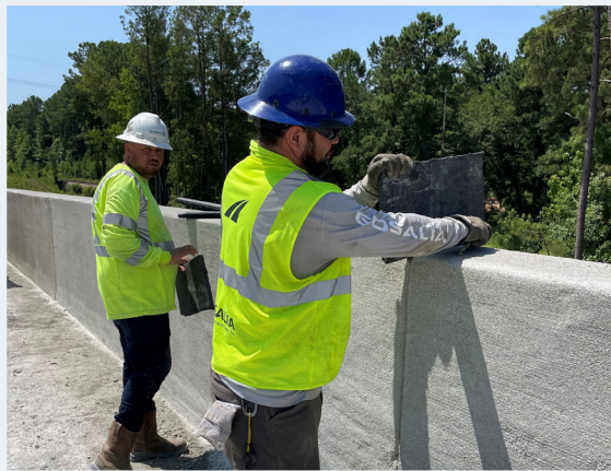
L – R: Luis Martinez and Oscar Hernandez, Gosalia Concrete Constructors, Inc., prepare to install expansion material in the concrete barrier.
