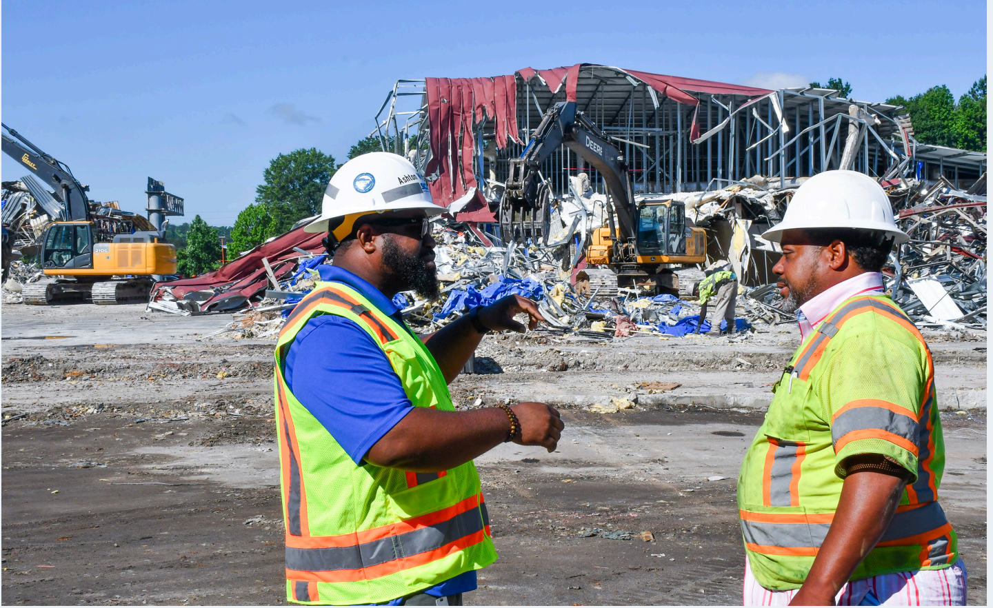
L-R: Ashton Williams, SCDOT Engineering Technician and Markus Corley, a co-owner of Corley Construction onsite at demolition on Browning Road which is part of CCR.
