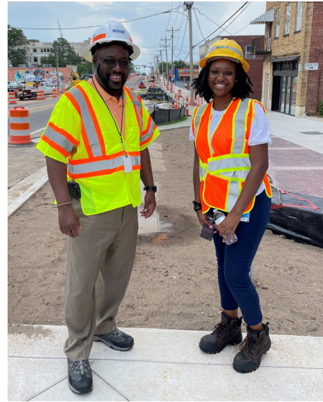
Greg Davis and Summer Intern Leila Kelly on-site at the South Main Street Project in Columbia.
