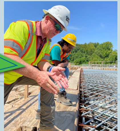
CCR RCE, Patrick Stinson, PE, CCM, DBIA of CDM Smith explains the purpose and related process of utilizing rebar/steel reinforcements on bridge steel structures at this CCR1 site along I-26 in Richland County.
