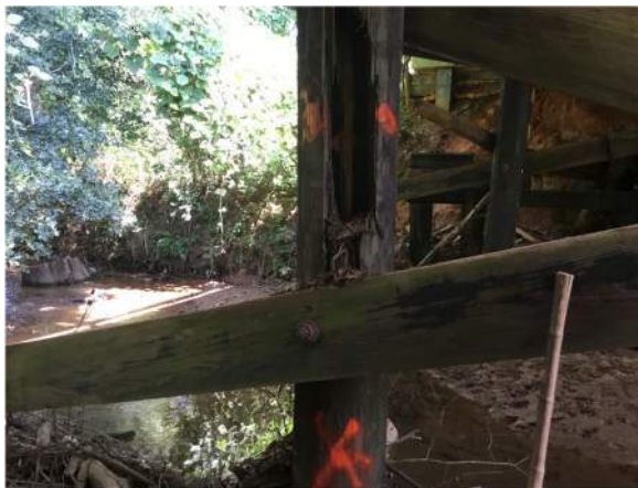
Figure 7.2 Exterior Pile with > 50% Decay, Drilling Not Needed (Critical Finding/A Flag per Figure O.3 in Appendix O)
