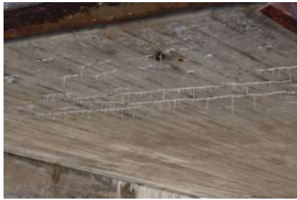
(1120 – Efflorescence/Rust Staining) Condition State 2
