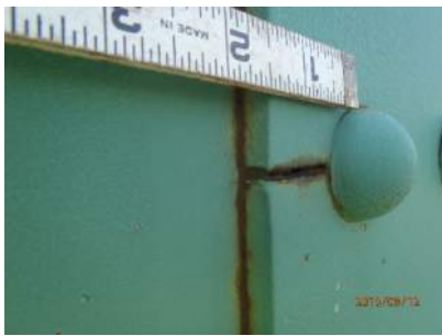
(1010 – Cracking) Condition State 2
