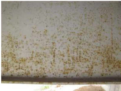
(1000 – Corrosion) Condition State 2
