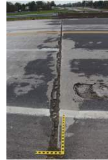
(2350 – Debris Impaction) Condition State 4
