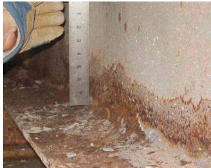
(1000 – Corrosion) Condition State 3
