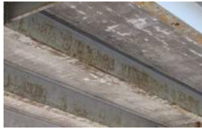
(3440 – Effectiveness) Condition State 3
