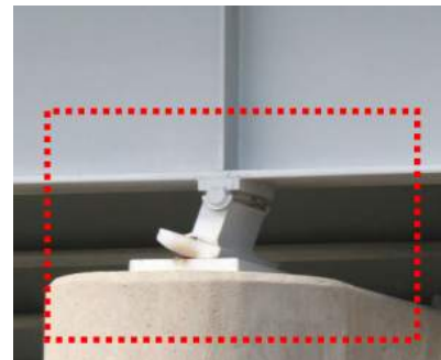
(2220 – Alignment) Condition State 3
