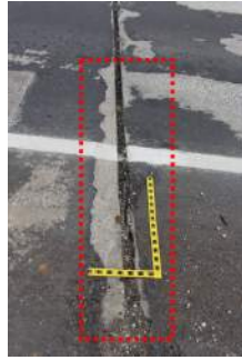
(2350 – Debris Impaction) Condition State 3
