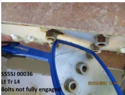
(1020 – Connections) Condition State 2
