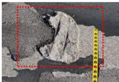
(1090 – Exposed Rebar) Condition State 2
