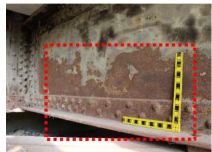
(3440 – Effectiveness) Condition State 4
