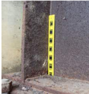
(3430 – Oxide Film Degradation) Condition State 3
