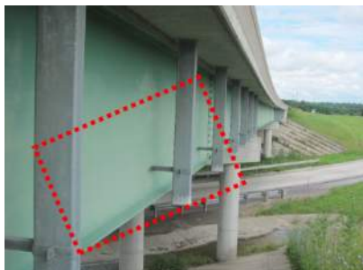
(3410 – Chalking) Condition State 2
