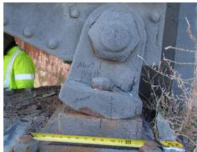
(2220 – Alignment) Condition State 2
