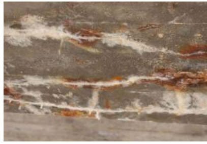
(1120 – Efflorescence/Rust Staining) Condition State 3
