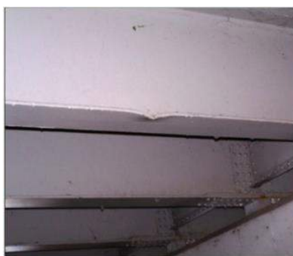
Condition State 2 (Damage)
