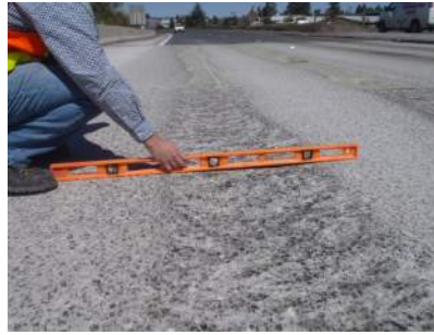
(1190 – Abrasion/Wear) Condition State 3
