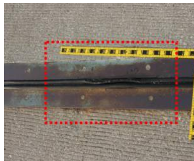
(2330 – Seal Damage) Condition State 3
