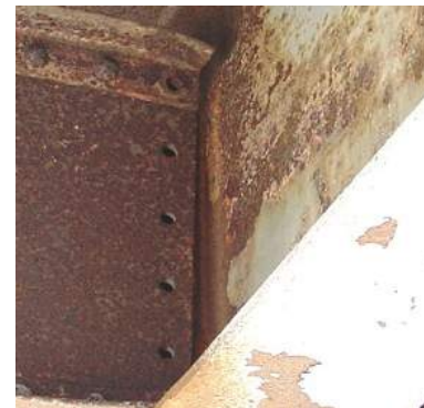
(1020 – Connections) Condition State 4
