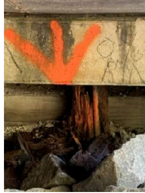
(1140 – Decay/Section Loss) Condition State 4
