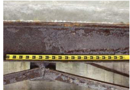
(3430 – Oxide Film Degradation) Condition State 3
