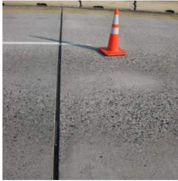
(1190 – Abrasion/Wear) Condition State 2
