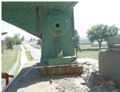
(2220 – Alignment) Condition State 1
