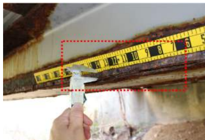
(1000 – Corrosion) Condition State 3
