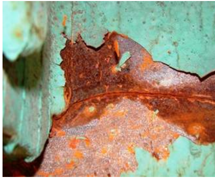
(1010 – Cracking) Condition State 3
