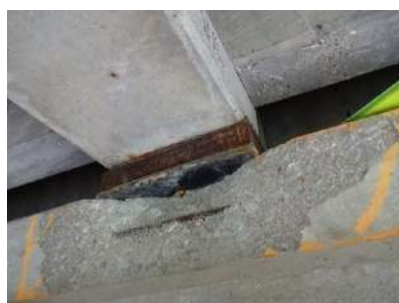
(2240 – Loss of Bearing Area) Condition State 3
