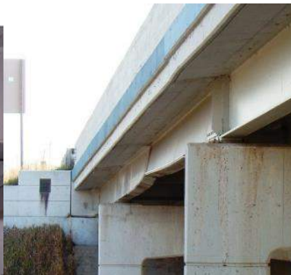
Condition State 3 (Damage)
