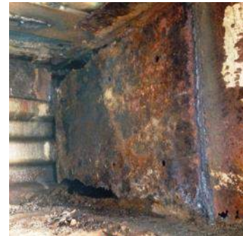
(1000 – Corrosion) Condition State 4
