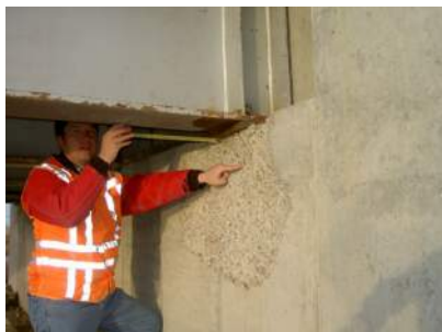
(2240 – Loss of Bearing Area) Condition State 2
