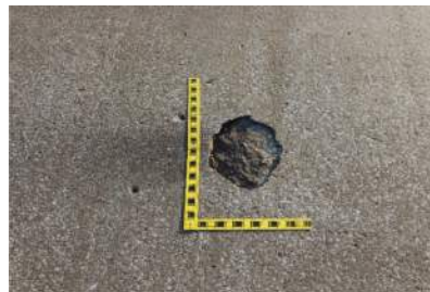
(1080 – Delamination/Spall/Patched Area) Condition State 3
