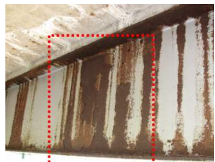
(3420 – Peeling/Bubbling/Cracking) Condition State 4
