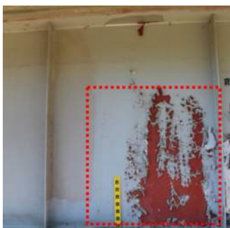
(3420 – Peeling/Bubbling/Cracking) Condition State 2
