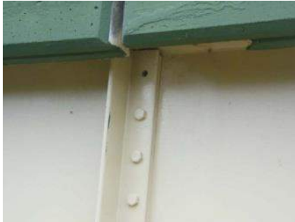
(1020 – Connections) Condition State 2
