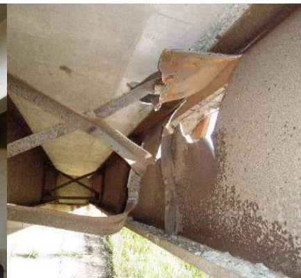
Condition State 4 (Damage)
