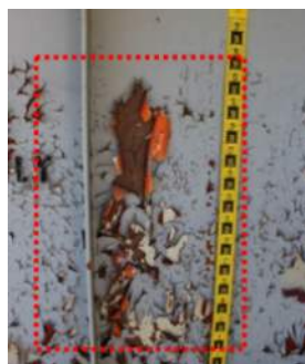
(3420 – Peeling/Bubbling/Cracking) Condition State 3
