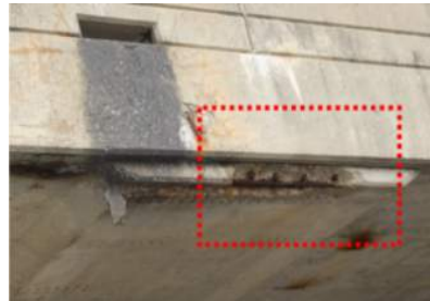
(1090 – Exposed Rebar) Condition State 3
