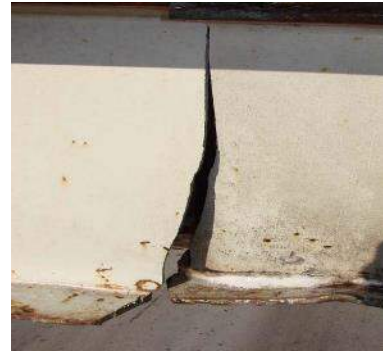
(1010 – Cracking) Condition State 4
