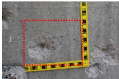
(1080 – Delamination/Spall/Patched Area) Condition State 2
