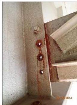
(1020 – Connections) Condition State 3
