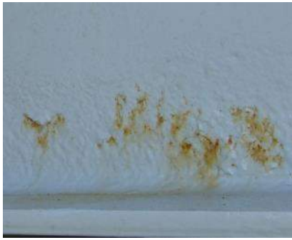
(1000 – Corrosion) Condition State 4
