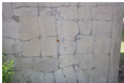
(1130 – Cracking/RC and Other) Condition State 3
