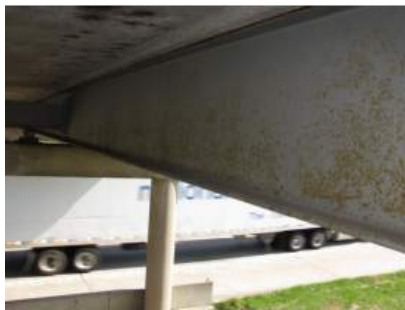
(3440 – Effectiveness) Condition State 2
