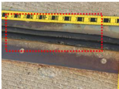
(2330 – Seal Damage) Condition State 2
