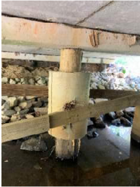
(1140 – Decay/Section Loss) Condition State 3*
