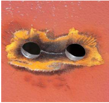
(1010 – Cracking) Condition State 2
