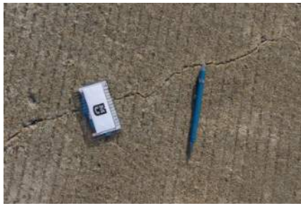
(1130 – Cracking/RC and Other) Condition State 2
