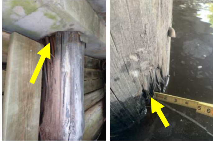
Figure 3.8 Shell damage to timber piling at or near the water line or at the pile cap, often caused by construction damage (left photo) or debris floating down the waterway at the waterline (right photo).
