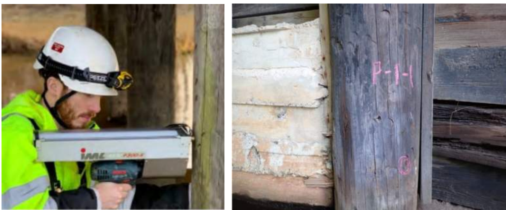
Figure 7.1 In field use of a resistance drill (left photo) and the field marking of a timber pile that has been drilled (right photo).
