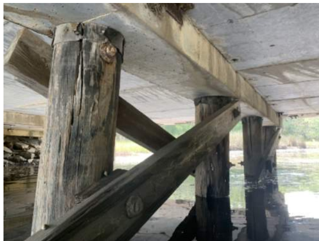
Figure 1.0 Example of a Timber Pile Bridge (Timber Piles under Reinforced Concrete Cap)
