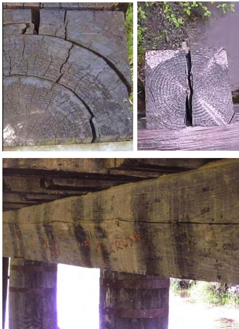
Figure 3.7 Timber members showing various types of deterioration. Top left shows ring shake. Top right shows severe through splits. Bottom picture is of a long horizontal split provides an opportunity for moisture passing through the timber deck to enter the cap, leading to substantial decay.
