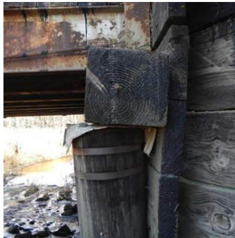
Figure 3.9 Severe misalignment of the timber pile and timber pile cap.
