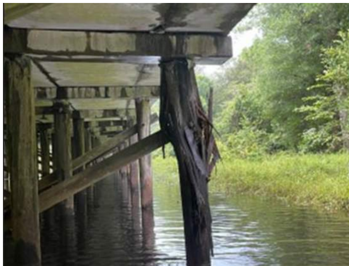
Figure 3.1 Failed timber pile due to internal decay of the pile at a cross-frame through bolt.
