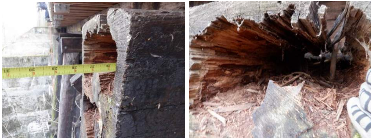
Figure 3.3 Localized collapse of a timber bent cap.
