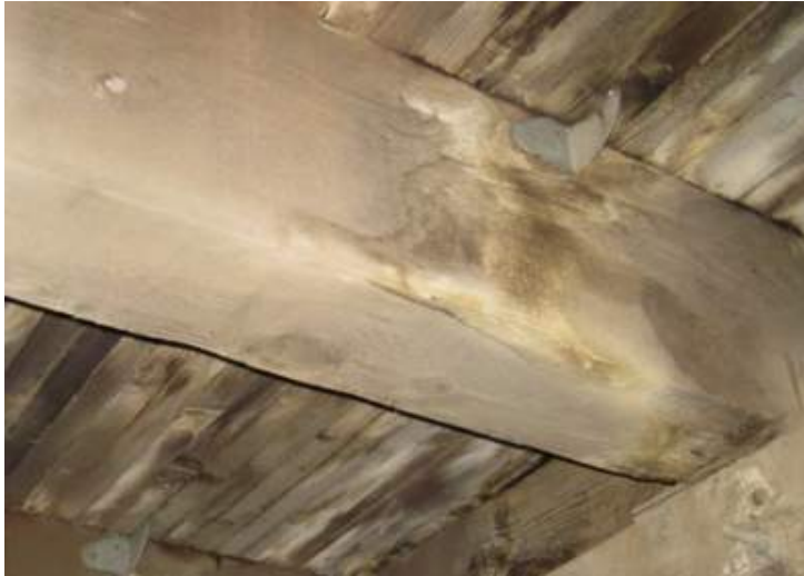
Figure 3.4 Water staining and discoloration caused by water that infiltrated through the wearing surface.
