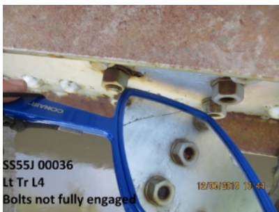
(1020 – Connections) Condition State 2
