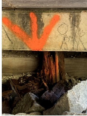
(1140 – Decay/Section Loss) Condition State 4
