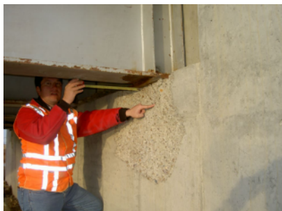
(2240 – Loss of Bearing Area) Condition State 2
