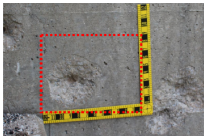
(1080 – Delamination/Spall/Patched Area) Condition State 2
