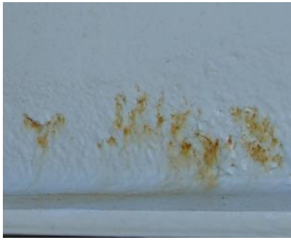
(1000 – Corrosion) Condition State 4
