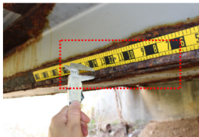
(1000 – Corrosion) Condition State 3
