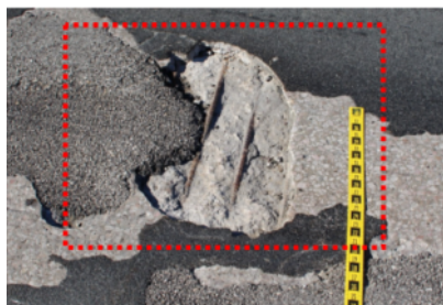
(1090 – Exposed Rebar) Condition State 2
