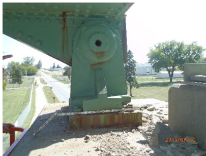
(2220 – Alignment) Condition State 1
