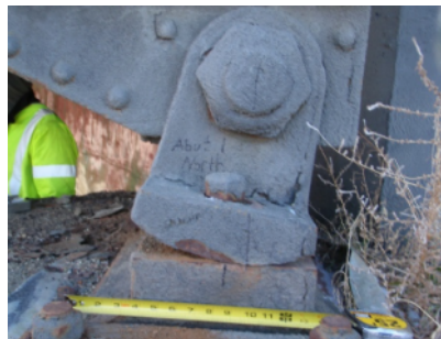
(2220 – Alignment) Condition State 2
