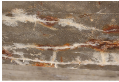
(1120 – Efflorescence/Rust Staining) Condition State 3
