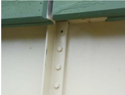
(1020 – Connections) Condition State 2
