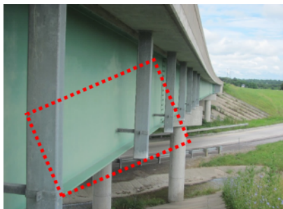
(3410 – Chalking) Condition State 2
