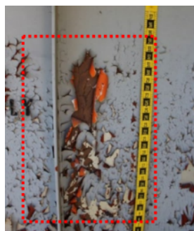
(3420 – Peeling/Bubbling/Cracking) Condition State 3
