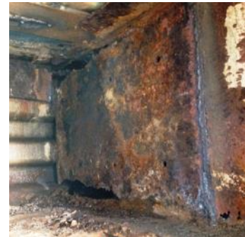
(1000 – Corrosion) Condition State 4
