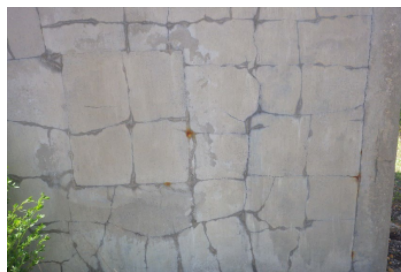
(1130 – Cracking/RC and Other) Condition State 3
