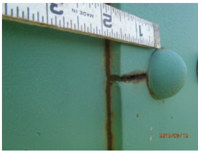
(1010 – Cracking) Condition State 2
