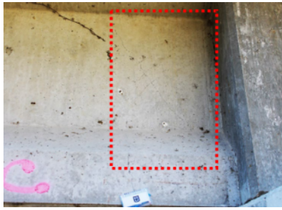
(1110 – Cracking/PSC) Condition State 2
