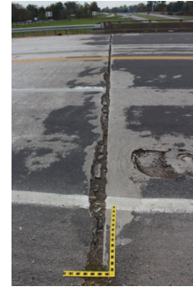
(2350 – Debris Impaction) Condition State 4
