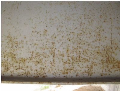
(1000 – Corrosion) Condition State 2
