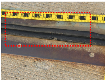
(2330 – Seal Damage) Condition State 2
