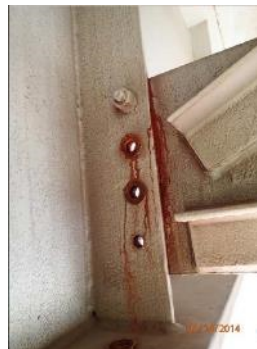
(1020 – Connections) Condition State 3
