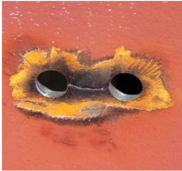
(1010 – Cracking) Condition State 2
