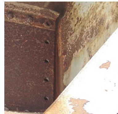
(1020 – Connections) Condition State 4
