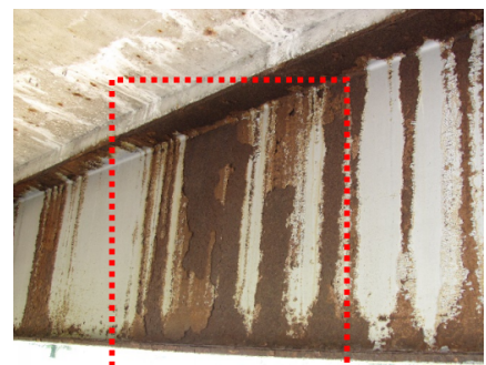
(3420 – Peeling/Bubbling/Cracking) Condition State 4
