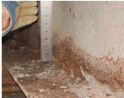
(1000 – Corrosion) Condition State 3
