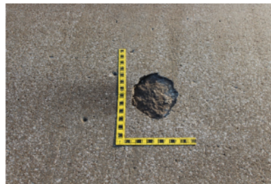
(1080 – Delamination/Spall/Patched Area) Condition State 3
