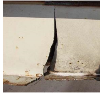
(1010 – Cracking) Condition State 4
