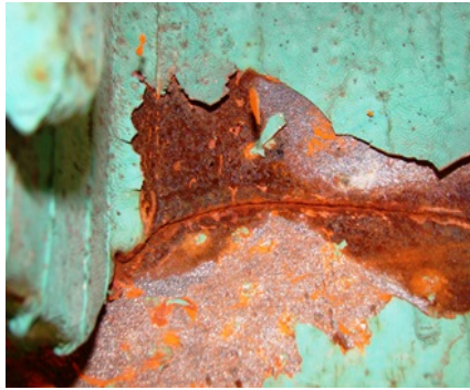
(1010 – Cracking) Condition State 3
