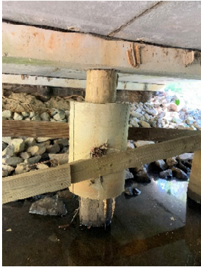
(1140 – Decay/Section Loss) Condition State 3*
