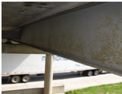
(3440 – Effectiveness) Condition State 2
