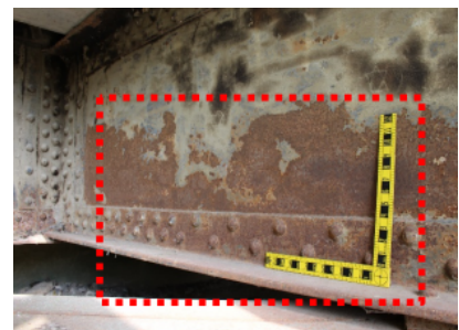
(3440 – Effectiveness) Condition State 4
