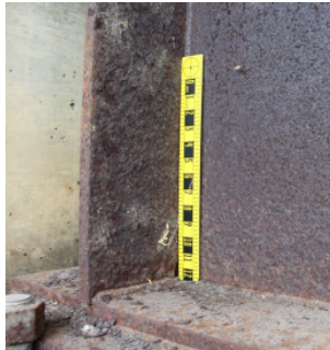
(3430 – Oxide Film Degradation) Condition State 3
