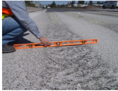
(1190 – Abrasion/Wear) Condition State 3
