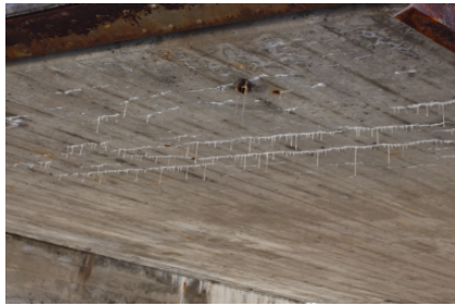
(1120 – Efflorescence/Rust Staining) Condition State 2
