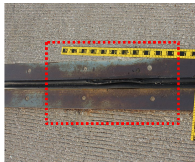
(2330 – Seal Damage) Condition State 3
