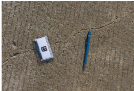
(1130 – Cracking/RC and Other) Condition State 2
