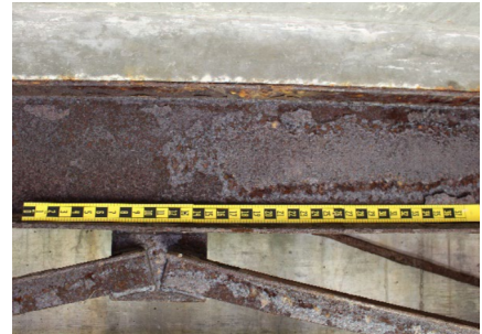
(3430 – Oxide Film Degradation) Condition State 3
