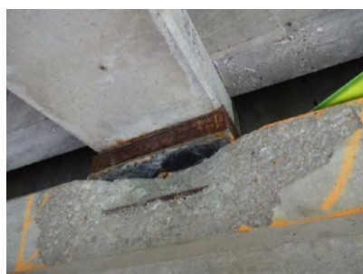
(2240 – Loss of Bearing Area) Condition State 3
