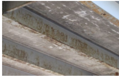
(3440 – Effectiveness) Condition State 3
