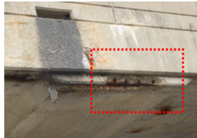
(1090 – Exposed Rebar) Condition State 3
