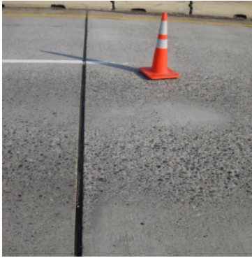
(1190 – Abrasion/Wear) Condition State 2
