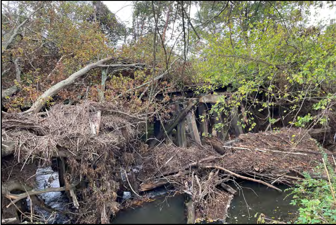
Figure 37. SHPO Site No. 6445, trestle bridge over Reedy River, looking northwest from Water Tower Apartments
