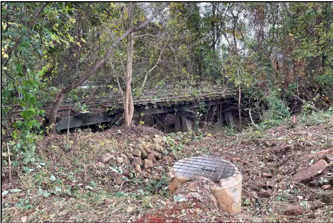
Figure 36. SHPO Site No. 6445, trestle bridge approach, looking northwest from Water Tower Apartments
