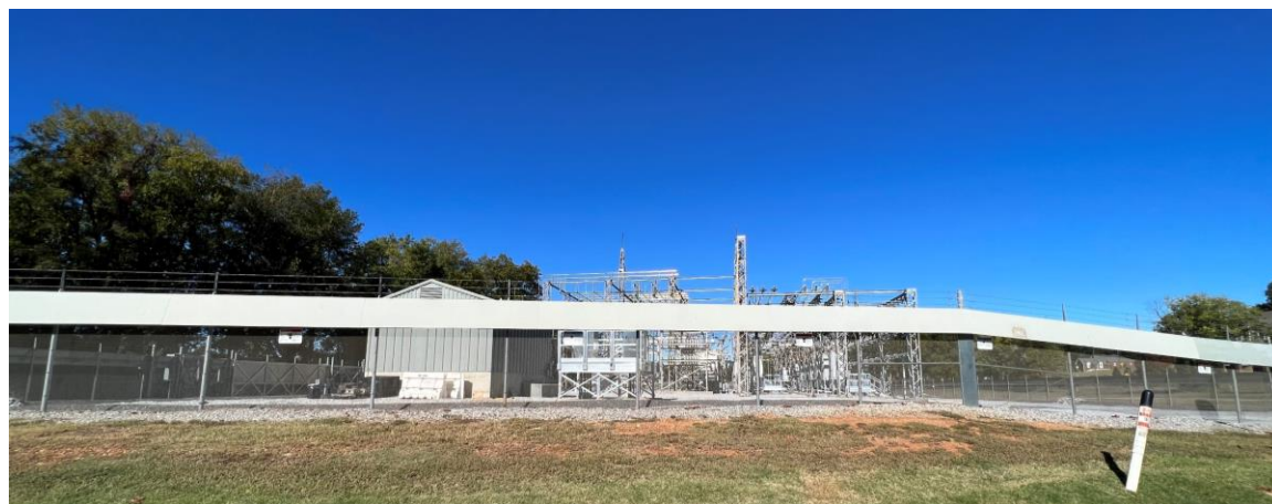
View of Parcels 11, 12, and 13, identified as "Transformer Yard" / Power Sub-Station / Gibbs Street Right-of-Way within EDR historical information, located at 299 S. Hudson Street within the Project Area. This potential PCB site is considered REC 13.
