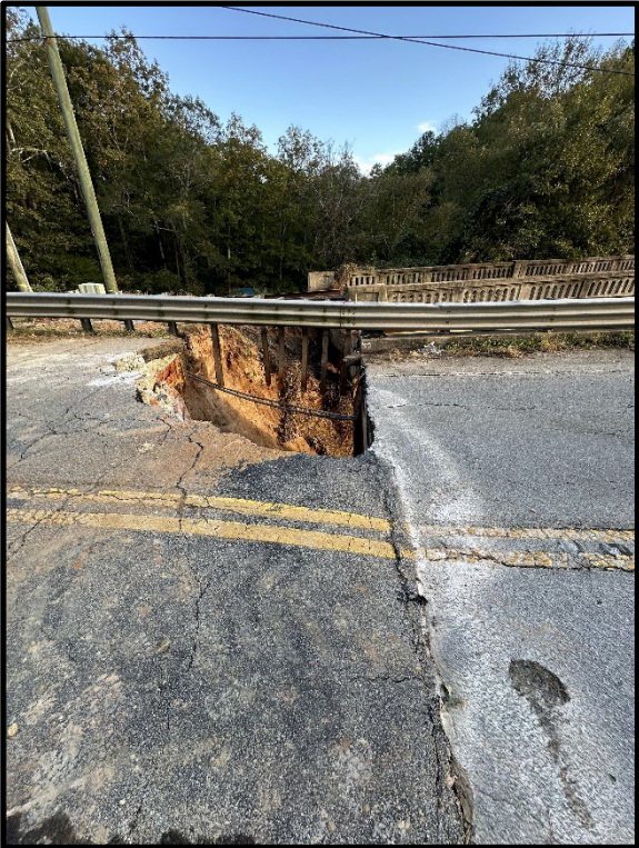
Eastbound Lane Damage
