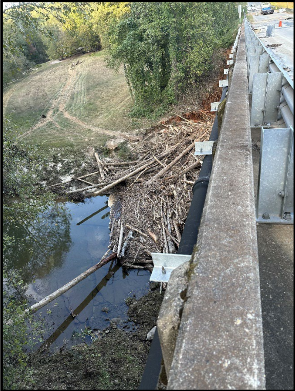
Debris Accumulation (North Side)
