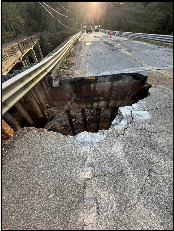
Eastbound Lane Damage
