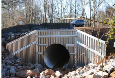
Use Pipe Wingwall
