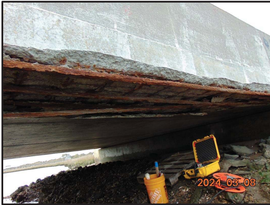
Photo 27: Spalling w/ Exposed Rebar Noted Throughout the Bridge Deck
