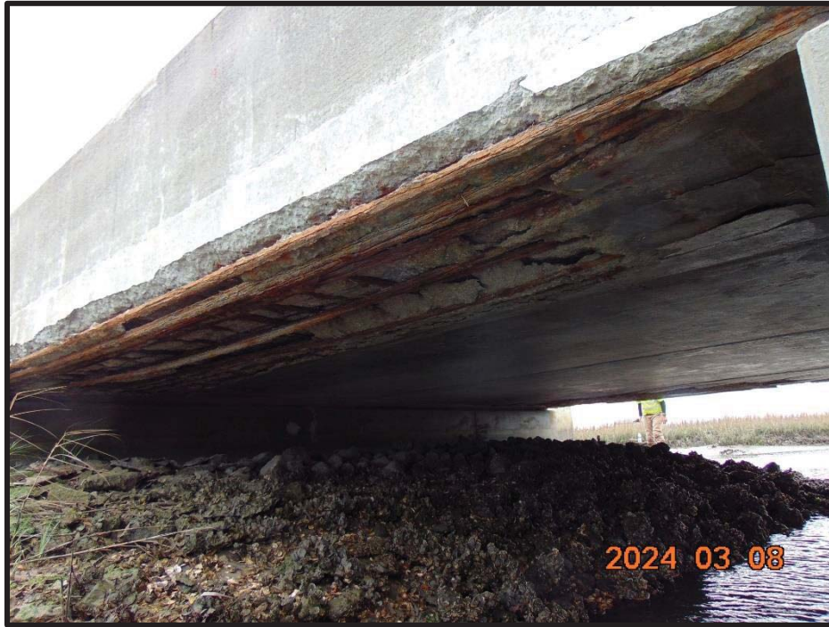
Photo 29: Spalling w/ Exposed Rebar Noted Throughout the Bridge Deck
