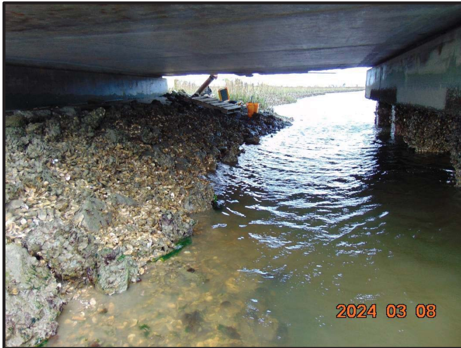
Photo 19: Scour Present Between Bents 3 & 4
