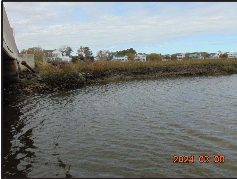
Photo 21: Erosion Present at Upstream Embankment
