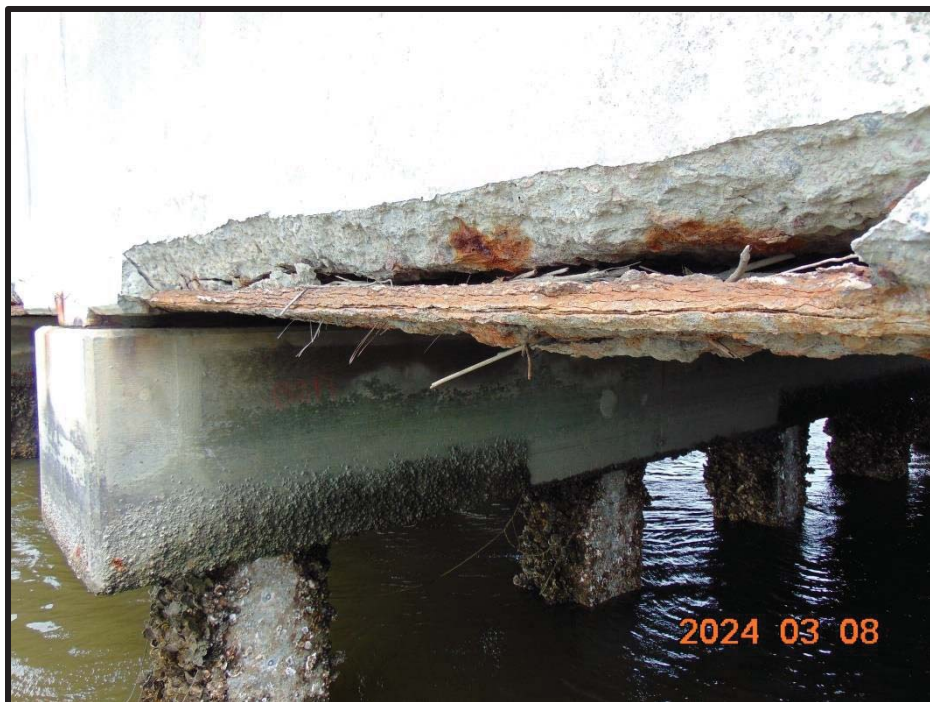
Photo 30: Spalling w/ Exposed Rebar Noted Throughout the Bridge Deck
