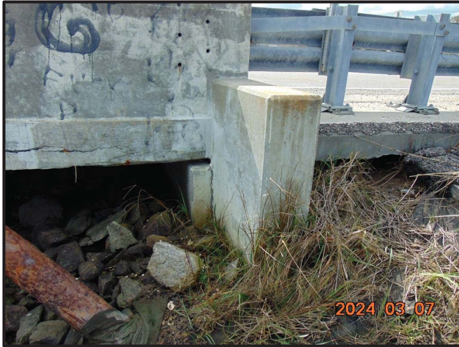
Photo 25: Erosion Present at Abutment 2
