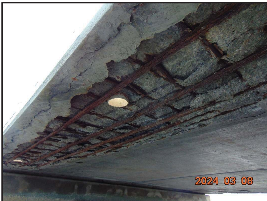
Photo 28: Spalling w/ Exposed Rebar Noted Throughout the Bridge Deck
