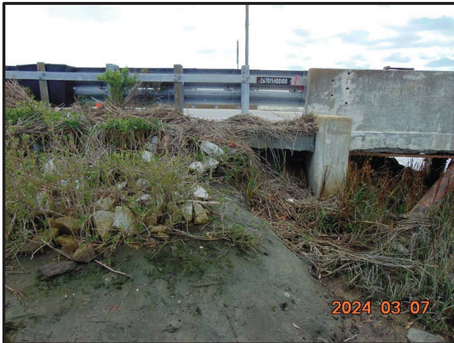
Photo 22: Erosion Present at Abutment 1
