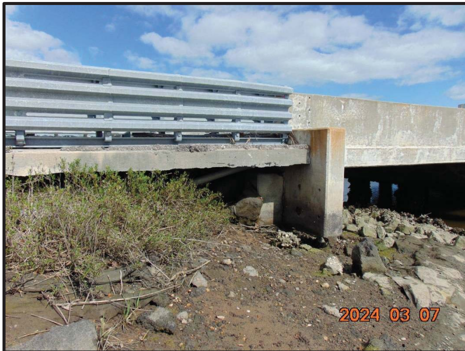
Photo 24: Erosion Present at Abutment 2
