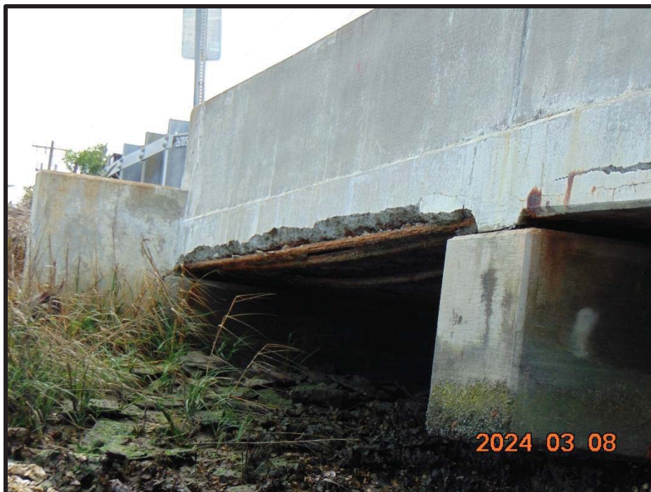
Photo 26: Spalling w/ Exposed Rebar Noted Throughout the Bridge Deck
