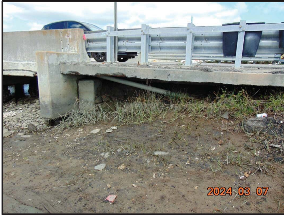
Photo 23: Erosion Present at Abutment 1
