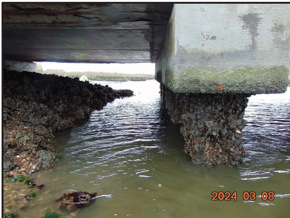
Photo 20: Scour Present Between Bents 1 & 2
