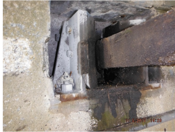
Photo 3 – Brake pads associated with the mechanical locking mechanism for the swing bridge.
