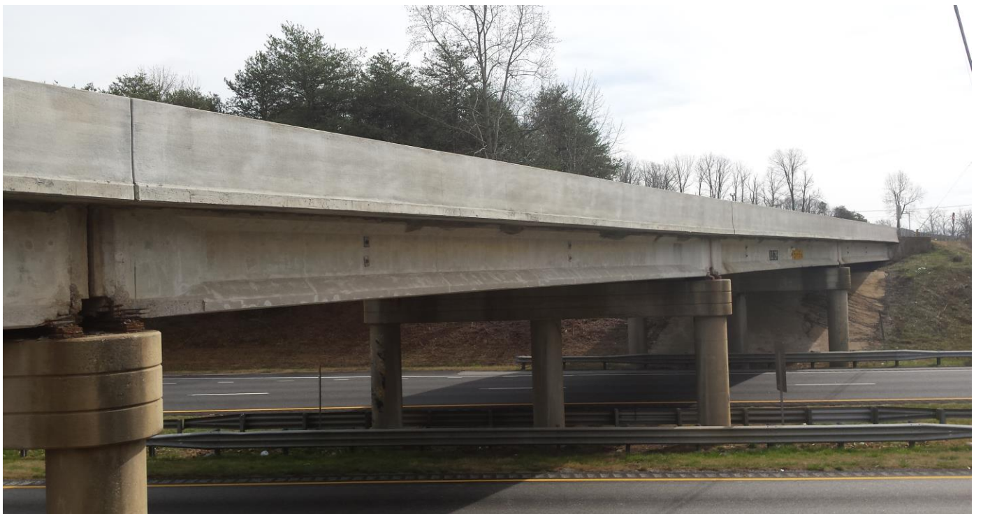
Photograph 2 –View of the side of the US- 29 (E. Cherokee St.) bridge at Exit 106 in Cherokee County, SC.
