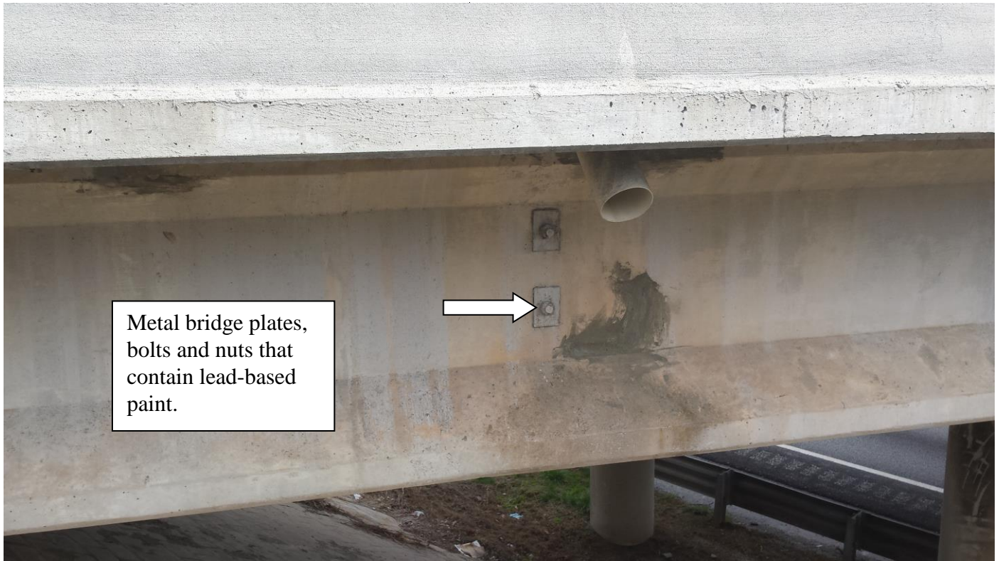
Photograph 3 – View of the metal bridge plates, bolts and nuts that contain lead-based paint.
