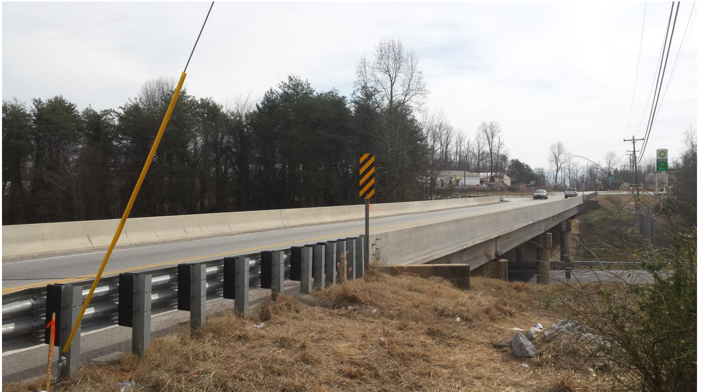
Photograph 1 – View of the top of the bridge structure at US- 29 (E. Cherokee St.) in Cherokee County, SC.
