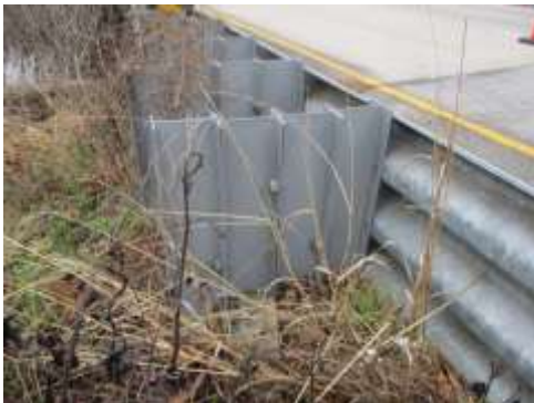
READING # 8, 9, 13 TYPICAL GUARD RAIL SUPPORT
