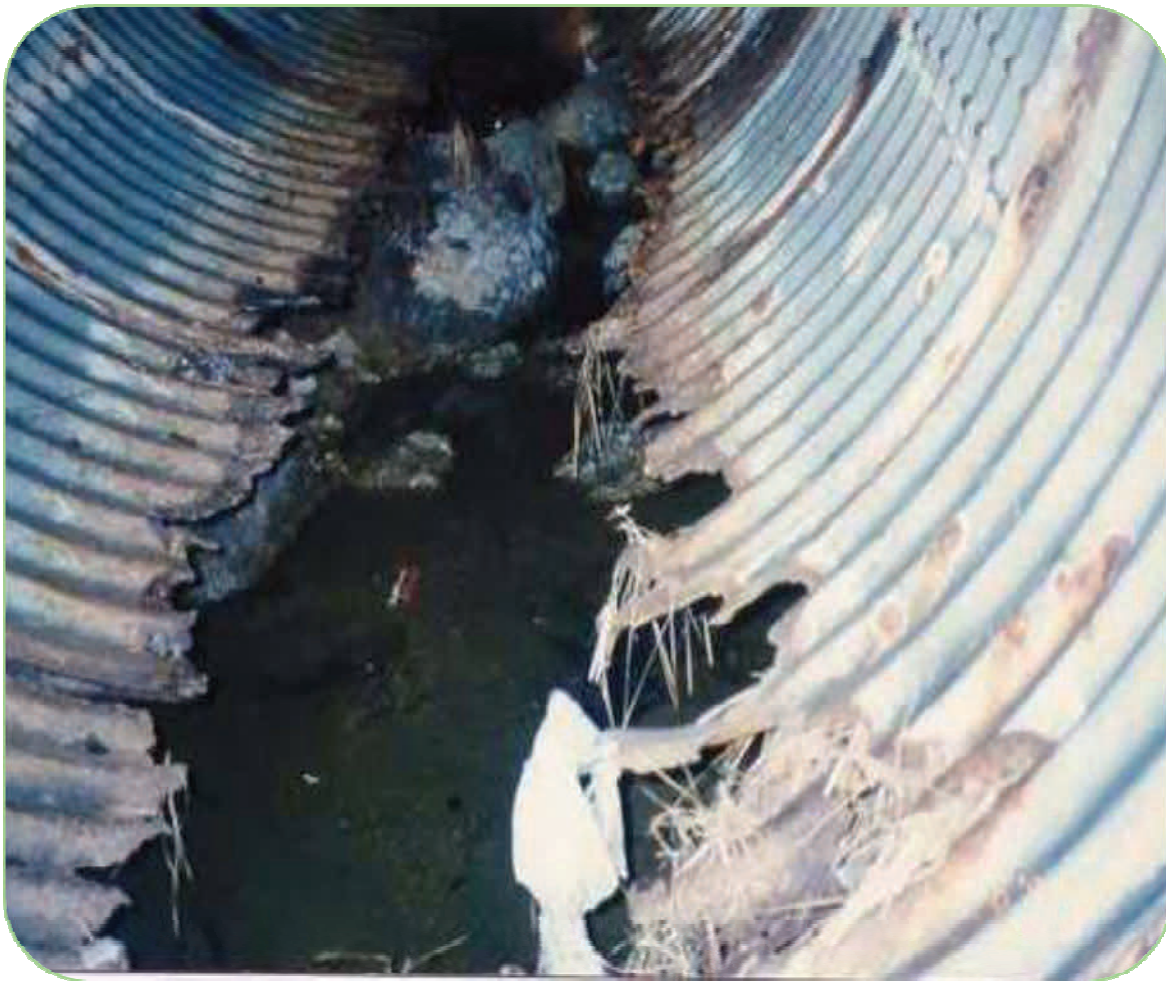
Severe Corrosion - Corrosion Rating 1
