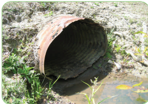
Old elliptical corrugated metal pipe
