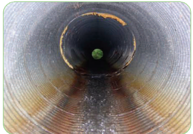
CMP Culvert with slight corrosion. Corrosion rating 5
