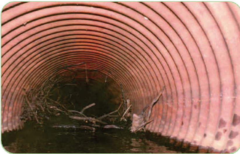
Culvert blocked with a Beaver Dam Blocked rating 2
