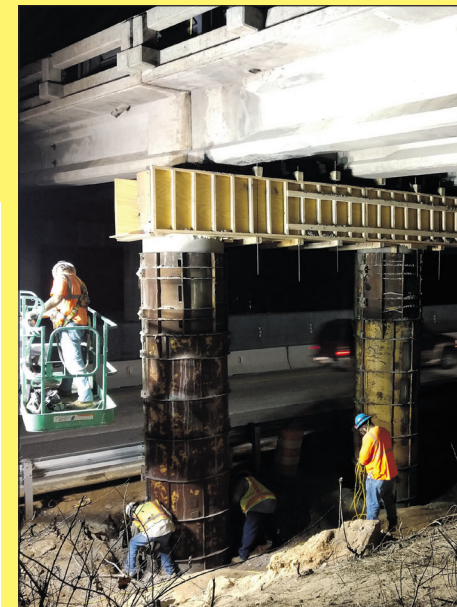
Crews made similar repairs to the Cedarcrest Road overpass in Lexington County.
