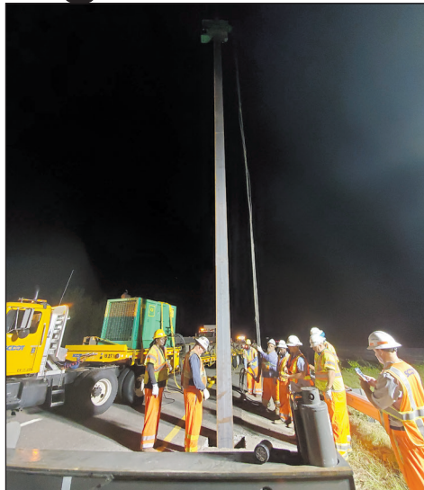
District Bridge and Richland Maintenance crews use a hydraulic hammer to drive a 50-ft steel pile into the ground to stop movement of a bridge slab on I-77.
