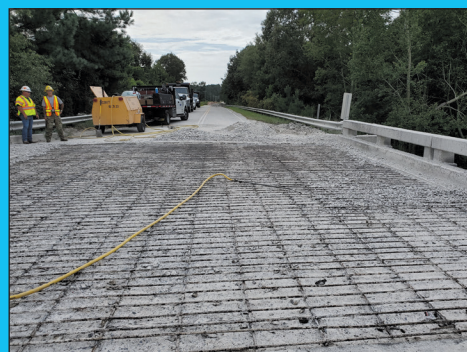
Kershaw Foreman Chris Team, and District Inspector Wil Pointer survey the work on the Old Charleston Bridge.
