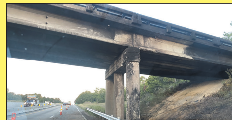
A truck hit and damaged the Cedarcrest Road bridge on I-26.
