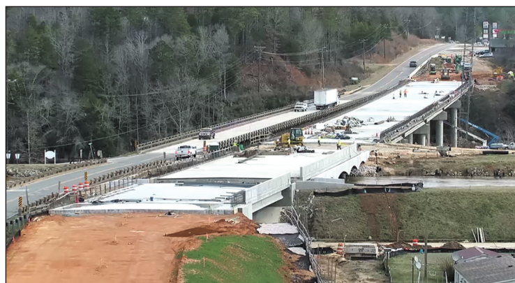
Four new bridges were built on a new alignment on S.C. 9 through the town of Lockhart.
