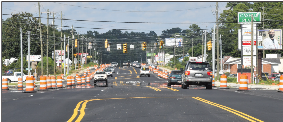
Repaving work is being completed on South Cashua Drive from 2nd Loop Road to Floyd Circle in Florence.
