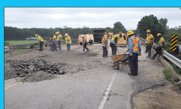
Lexington and Kershaw Maintenance Crews chip away deteriorated asphalt and concrete layers from the Old Charleston Road bridge over I-20 in Lexington County.
