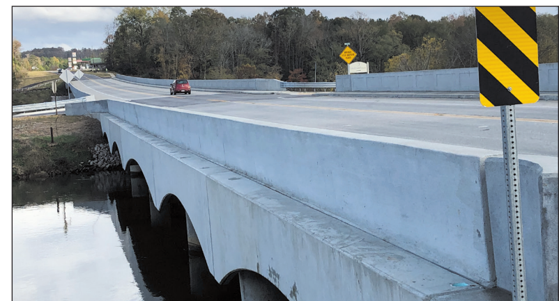
RIGHT: The project included a new bridge over the Broad River Canal.
