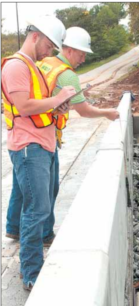
District 3 Bridge Inspectors Brandon Avant, left, and Vince Wade inspect a bridge on Highway 201 in Spartanburg County near Woodruff. Inspections are important for new and old bridges.
