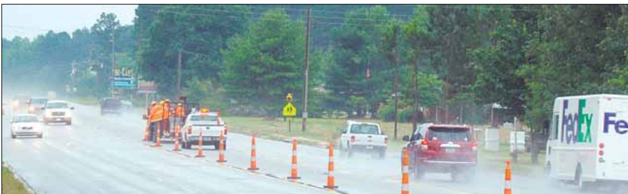
On June 5, District 5 participated in the Emergency Lane Reversal as part of the hurricane preparedness plan. Marion and Horry Maintenance, with assistance from other counties, put cones on Highway 501 and other emergency exit routes to make sure the process operated smoothly.
