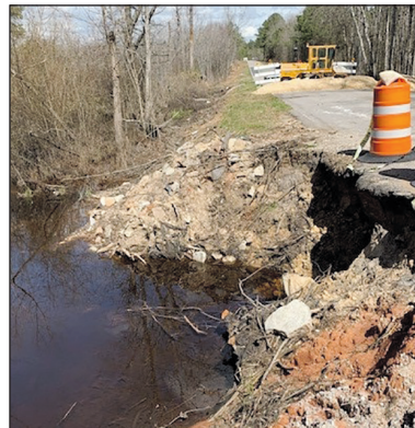
BEFORE: The failure is shown here on Spencer Road in Sumter County.
