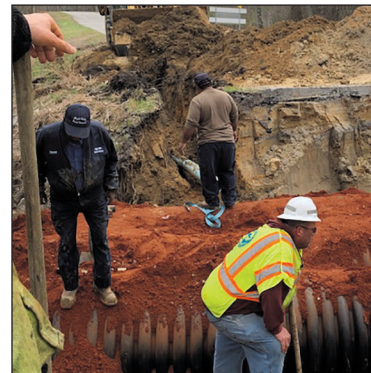
Sumter Safety Officer Hugh Hood checking work in the trench as two workers from High Hills Rural Water assist with relocating their utility line around the new pipes.
