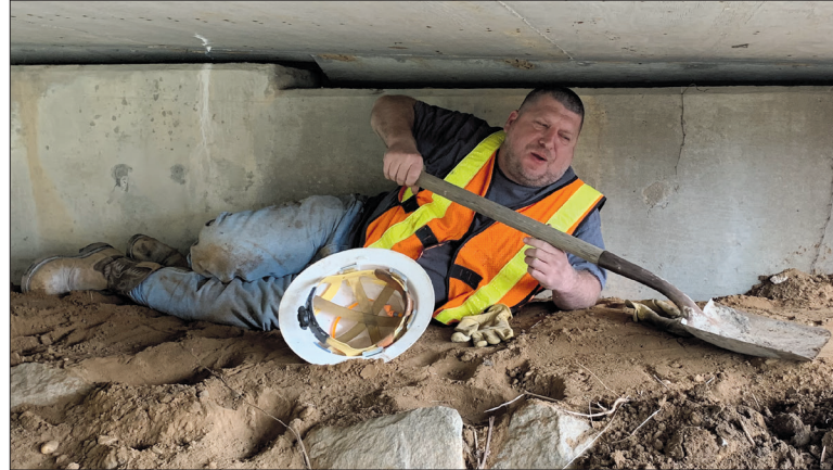
Harold Ballard is in a tight spot under I-20 in Kershaw County making room for the crew to work on repairs of a bridge slab that moves under traffic loads.
