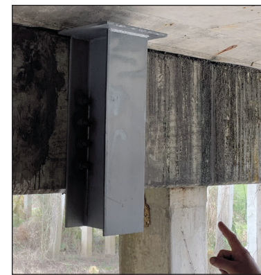
A further insurance to the slab-pinning, the opposite end of the "walking slab" has saddles epoxy-anchored to support any additional movement that should not occur after the repair is completed.
