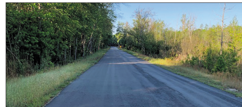
AFTER: The finished project replaced pipes, moved utilities and put up barriers to prevent beaver damage.
