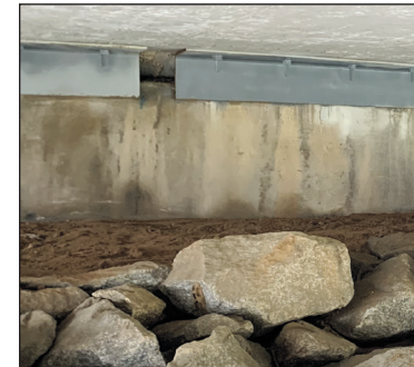
Each section of angle iron pinning the bridge slab to the bridge cap weighs in excess of 275 pounds. They are fastened to the bridge slab with many epoxy-set bolts in a designed pattern.
