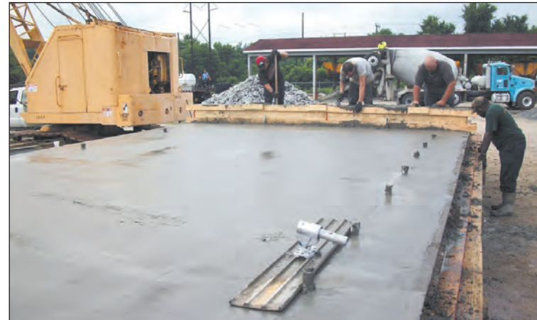
From left to right: Thomas Nesbitt, Chris Napper, Benji Catoe, and Robert Oliver (retired) put the finishing touches on a series of bridge panels that together make one span. The panels are cast together so when split apart for transport they will fit perfectly back together.
