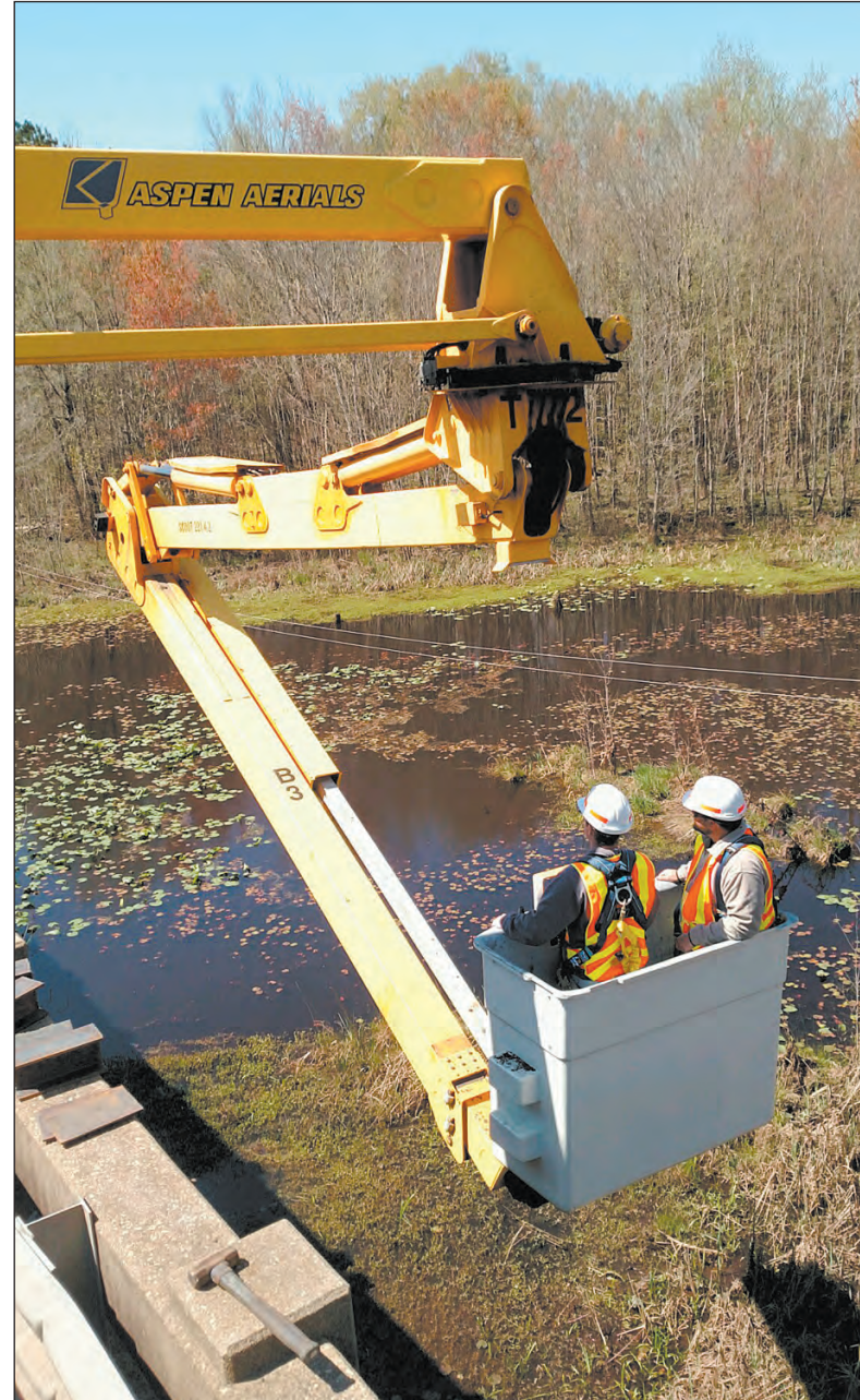
District 5 Bridge Inspection employee Mitch Elmore trains new employee Jeffrey Matthews on the operation of the snooper truck as they go under a bridge on U.S. 1 in Marlboro County to inspect repairs.
