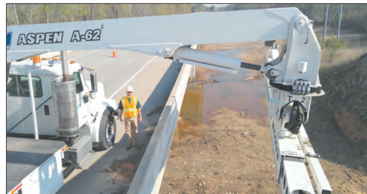
Brian Cobb looks on as Will Pointer goes "over the edge and under the deck" to inspect a newly-constructed bridge on U.S. 601 in Richland County.
