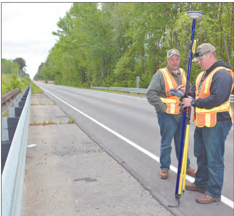
Bert Shumpert, left, and John Magni of Preconstruction Surveys set control points on the Bluff Road bridge over Back Swamp on April 15.
