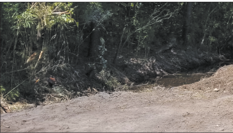
AFTER: The drainage ditch is able to move water faster with less potential for flooding. Employees from across the state participated in the effort.
