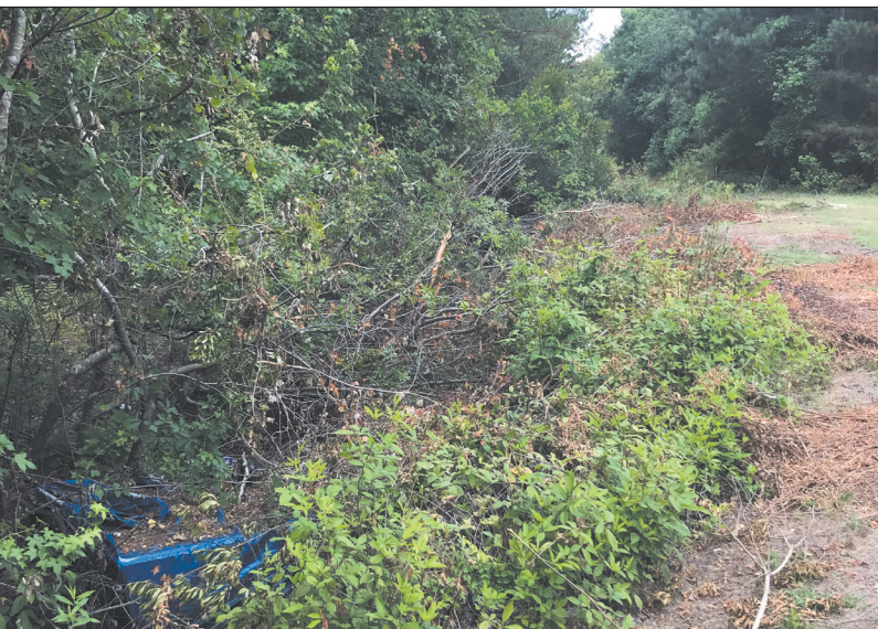
BEFORE: After years of neglect and litter accumulation, this major drainage ditch in Nichols is clogged and its drainage ability has been reduced.
