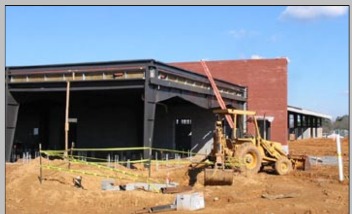
York Maintenance will have a new facility to call home soon. The Complex is located on Ogden Road in Rock Hill on a 22-acre tract. Construction on the $5 million dollar facility began in August 2005 and should be completed by July 2006.
