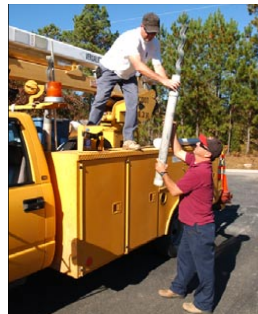
Del McCollum, left, and Brian Clack load supplies before heading out to repair traffic signals in Florida.
