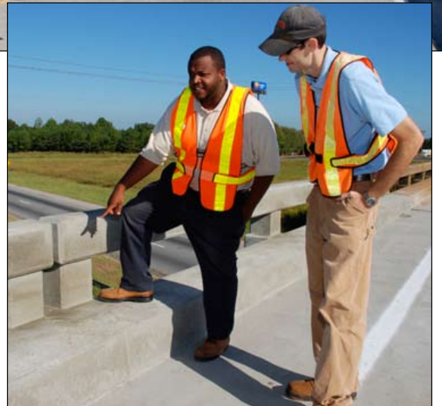
RIGHT: Asst. Newberry RCE Shawn Salley, left, and Newberry RCE Matthew Shealy check the new railings on the repaired bridge in Laurens County. Levi Cumalander and Tim Connelly, not pictured, of Newberry Construction were the night inspectors on the project. John Burnette, inset above, is the District 2 Bridge Inspector.
