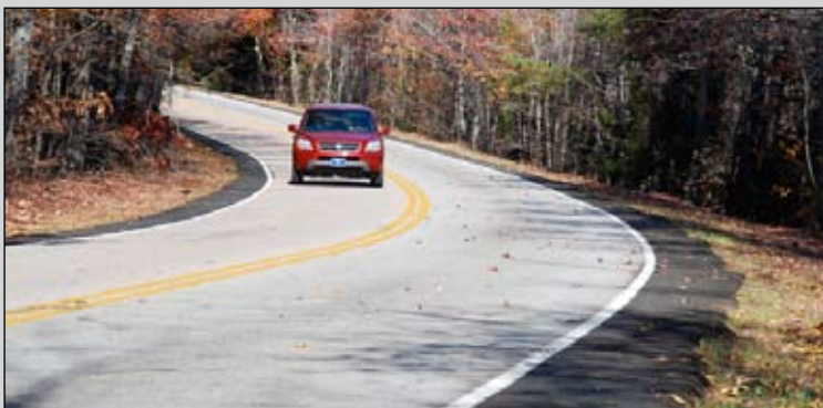
2-foot paved shoulder widening on Old White Horse Road in Greenville County
