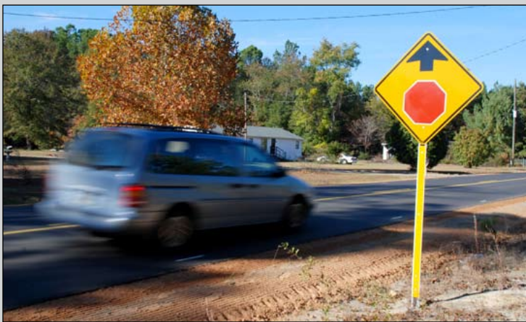
Reflective sign, new paving, striping and shoulder work on Stagecoach Road in Florence County
