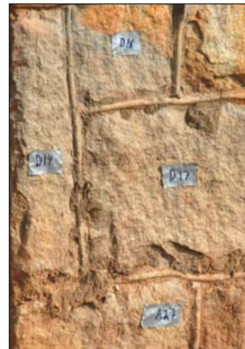
Each piece of the stone structure was numbered and labeled with duct tape. If the structure cracked or fell apart, the numbered labels would help put it back together.
