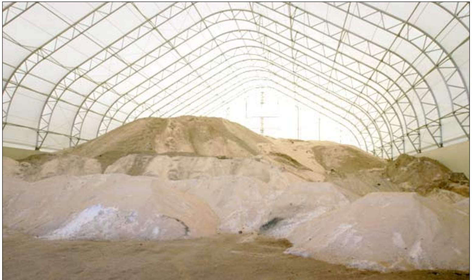
The "Mega Salt Dome" on Shop Road stores 10,000 tons of salt for use in inclement weather. The facility has concrete walls along the base with a domed PVC roof.
