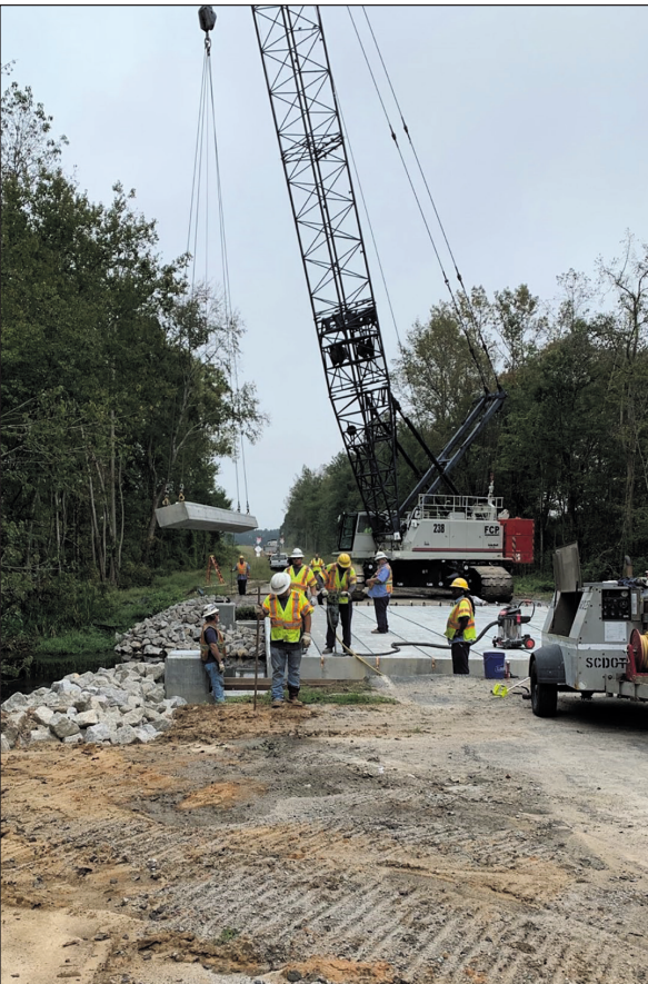
The District 1 Bridge Crew sets the last bridge panel with help from Kershaw and Lee Maintenance. This bridge is on Mary McLeod Bethune Road over Long Branch Creek in Lee County.
