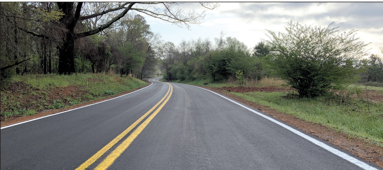
This image shows the finished surface course on a cement reclaimed base on Clinkscales Road in Anderson County.
