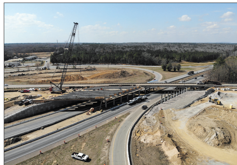
The Peak exit (Exit 97) is part of the Midlands Connection project on I-26. This exit will be a future diverging diamond interchange.
