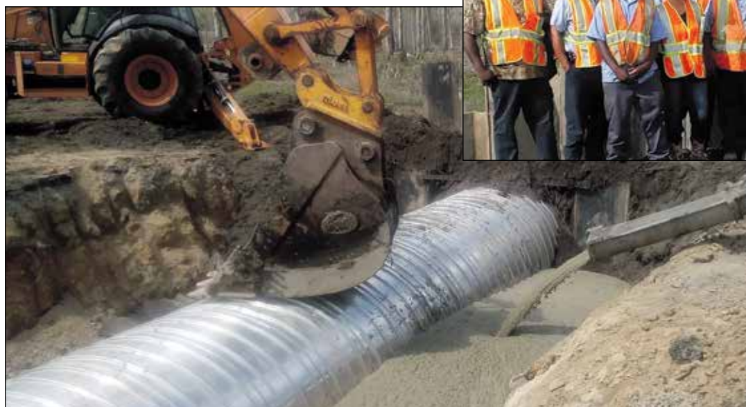
Flowable concrete fill is placed into the hole to solidify the pipe installation. The trackhoe bucket was used to help keep the pipe from floating up inside the fill.
