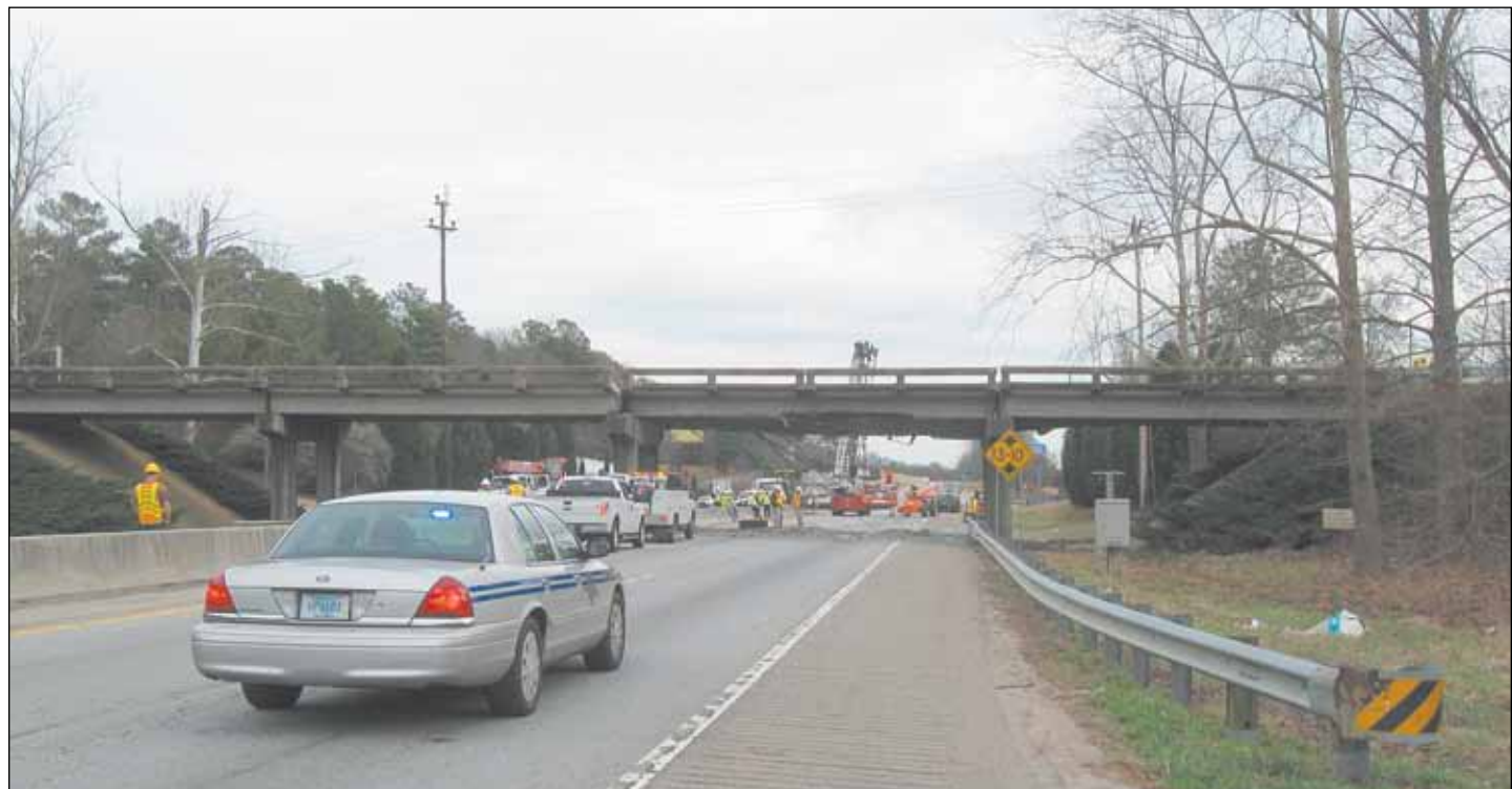
I-585 was closed for a day after a truck hit the California Avenue overpass and caused it to shift several feet. SCDOT crews worked through the night to demolish the damaged span by rush hour the next day. See more photos on page 26.
