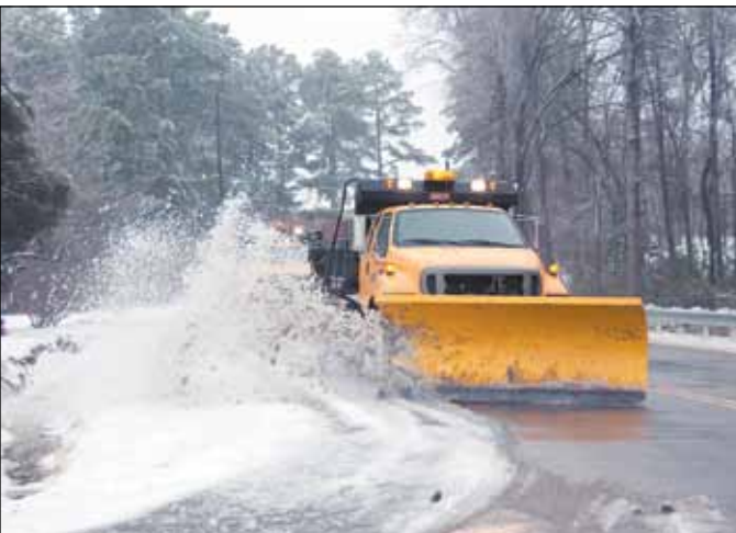
ABOVE: Richland Maintenance employees work in tandem to clear ice and snow from Highway 21.
