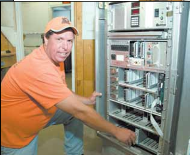
Jim Strickland from District 1 looks in a traffic signal cabinet. The traffic signal cabinet is the 'brain' of every intersection with signals.
