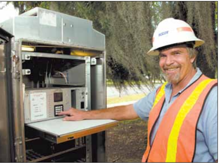
Benny Inman, of the District 5 Traffic Signal crew, checks a signal box at the intersection of a newly repaired traffic signal in Marion.
