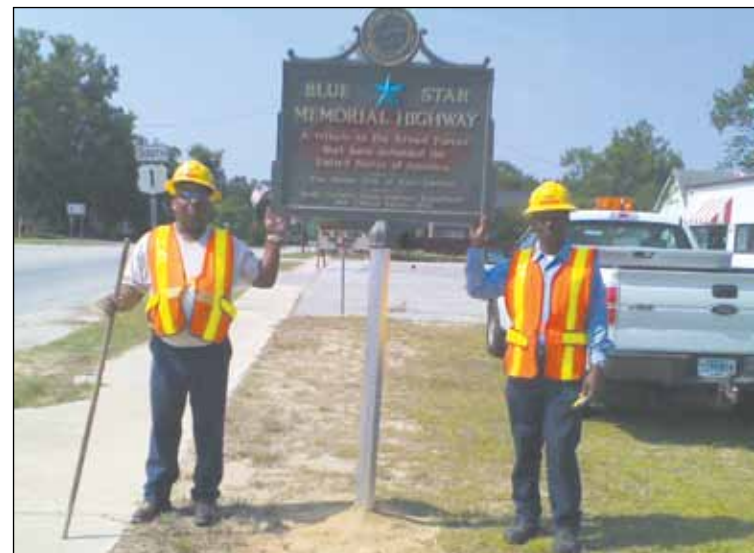
Chesterfield SCDOT employees RD Ratliff, left, and Donnie Rivers put the restored Blue Star Marker in place.
