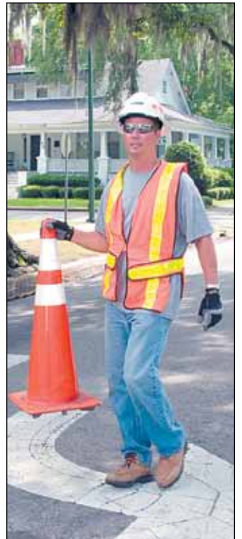
District 5 Traffic Signal crew member Chad Herlong picks up and loads traffic cones onto the truck after the job is completed in Marion.
