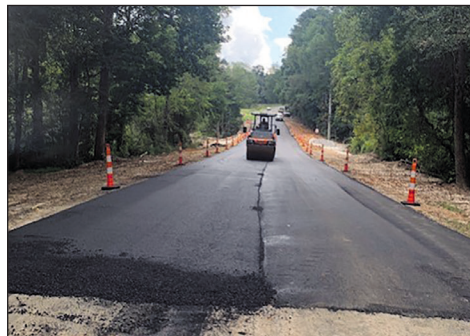
Lexington Maintenance installs initial asphalt surface to open Boiling Springs Road to traffic. The final resurfacing will be done later by contractors.
