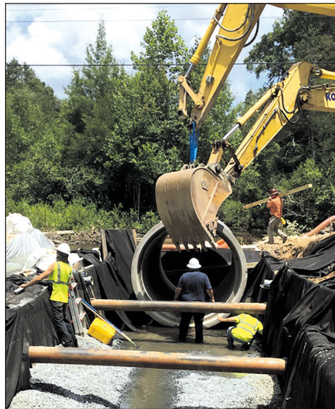
The contractor's successful installation depended on a lined diversion ditch and integrated trench boxing methods.
