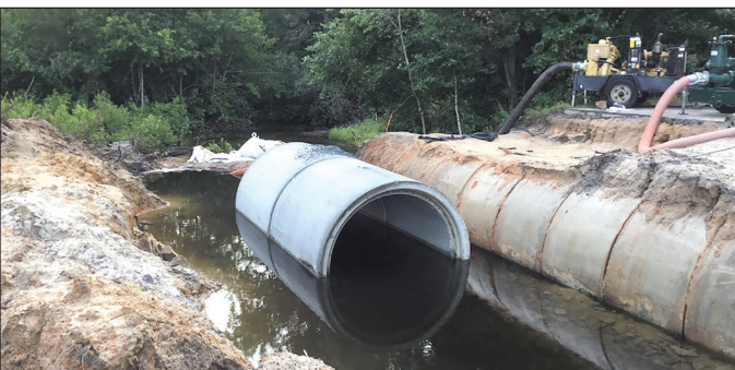
The contractor's first attempt to install new pipe was flooded by heavy rains.
