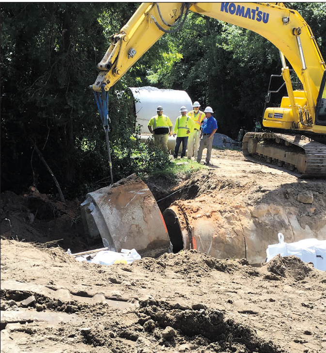
Four-foot long sections of 84-inch reinforced concrete pipe are removed for replacement.
