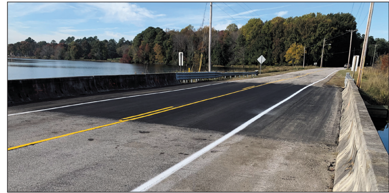
The Beauty Spot Road bridge over Lake Paul Wallace was repaired by District 5 employees.
