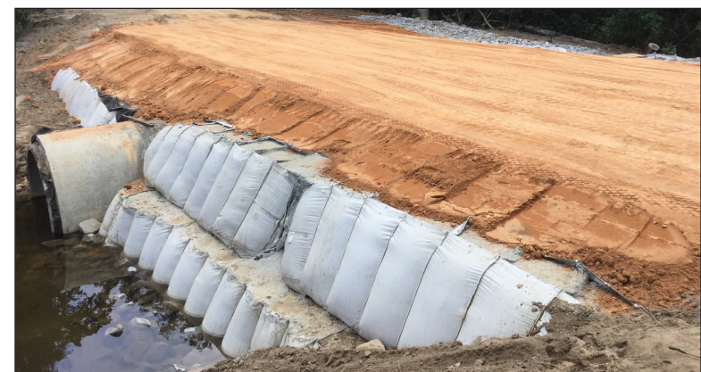
A patented concrete bag retention wall was installed and final dirt grade was done by Lexington Maintenance.
