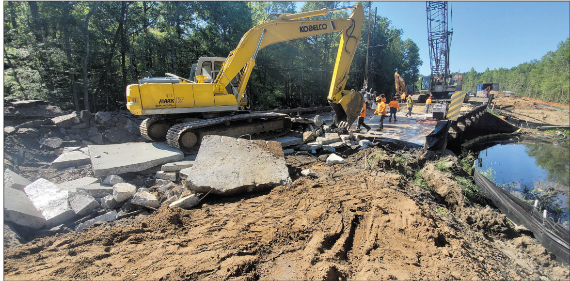
BEFORE: Crews demolish the original bridge that was load restricted and structurally deficient.
