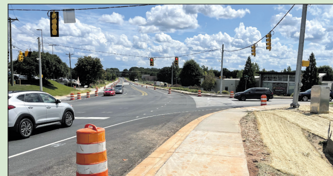
Here, work progresses at the corner of Scuttletown Road and Adams Mill Road which is part of the Woodruff Road widening project.
