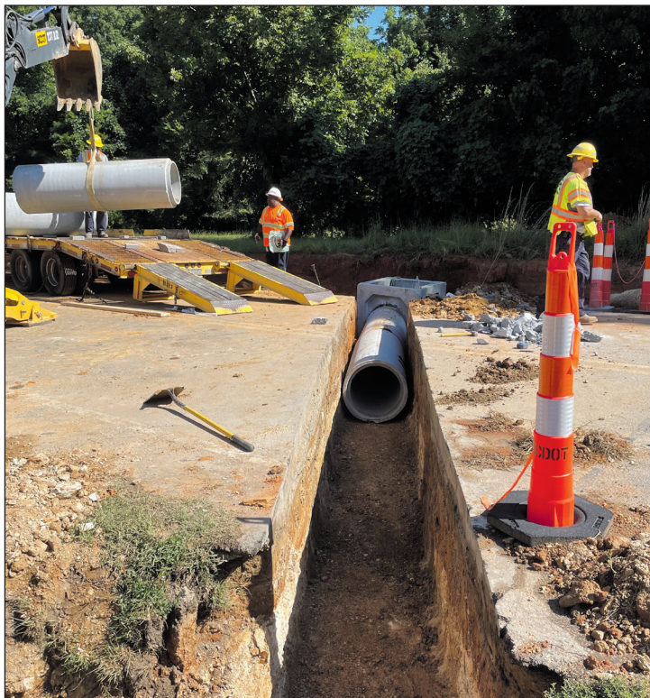
Lexington Maintenance crews install a 24-inch concrete pipe to alleviate a flooding issue on Calks Ferry Road.
